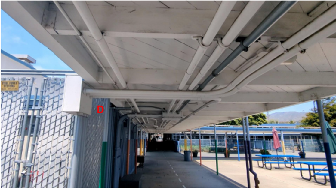
Document exposed conduit(s) entering electrical yard and adjacent building to remain
