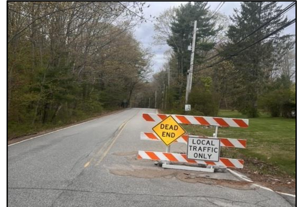
Road Closure: Scottow Hill Rd at Two Rod Rd due to culvert failure
