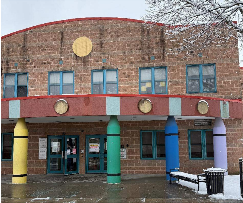
Front entrance access exhibits visible staining on masonry surfaces.
