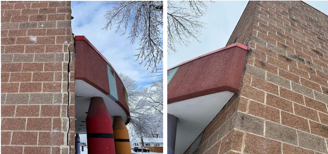
Front entrance canopy exhibits structural movement, resulting in separation of the veneer masonry from the CMU backup wall.
