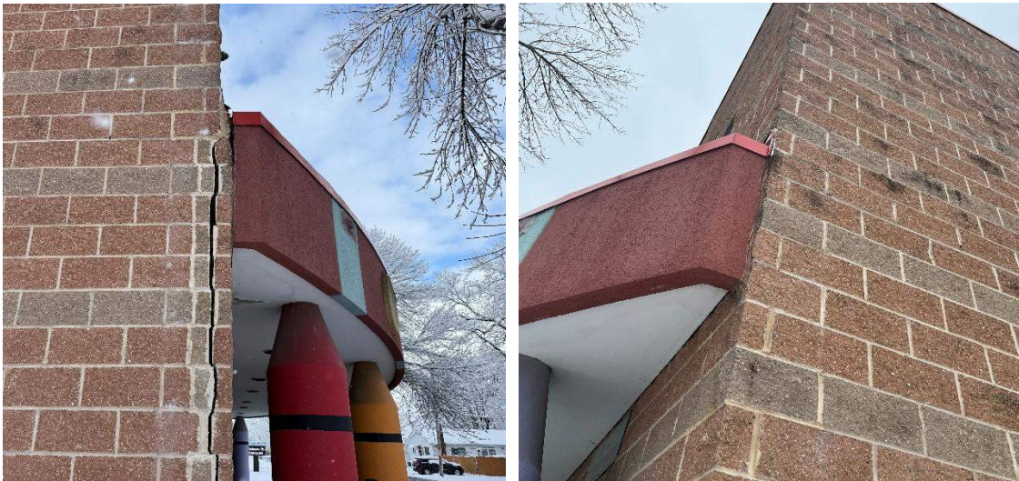
Front Entrance Canopy structural movement
