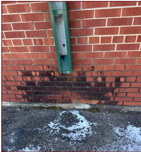
Moisture building has stained & discolored the lower brick masonry. Improper drainage has also caused surface deterioration and residue on the pavement at the base of the wall.
