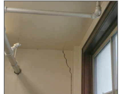
Water infiltration has caused structural cracking.
