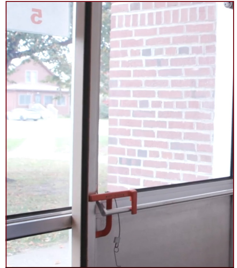
Exterior doors no longer seal and lock so additional locking devices need to be added.
