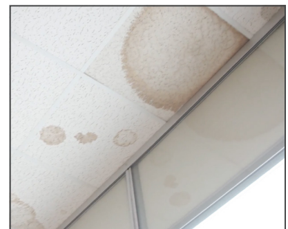
Failing roof sections have caused leaking and ceiling damage.
