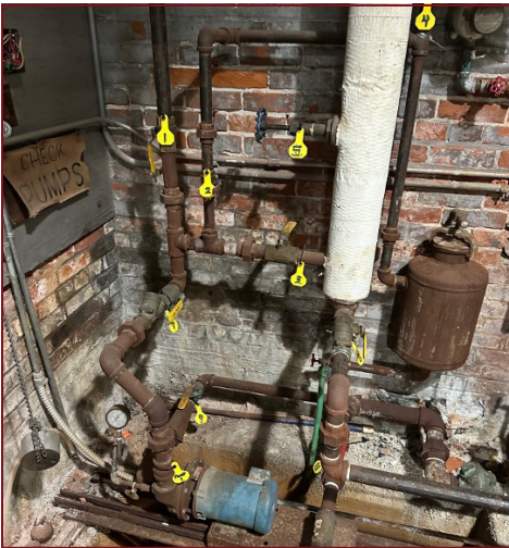
The mechanical room contains an outdated hydronic heating system with exposed piping, valves, a circulation pump that are outdated and corroding.
