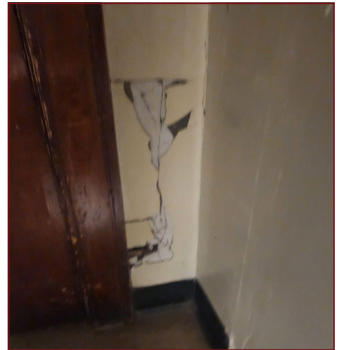
Interior wall surfaces are deteriorating.
