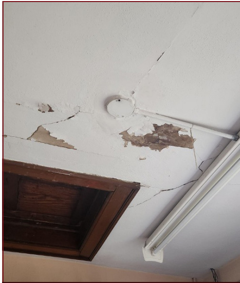
The ceiling has significant water damage.
