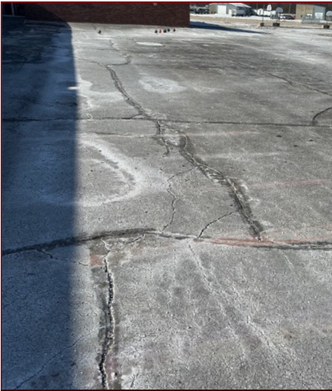
The elementary school back parking lot is deteriorating, with cracked pavement and drainage issues.
