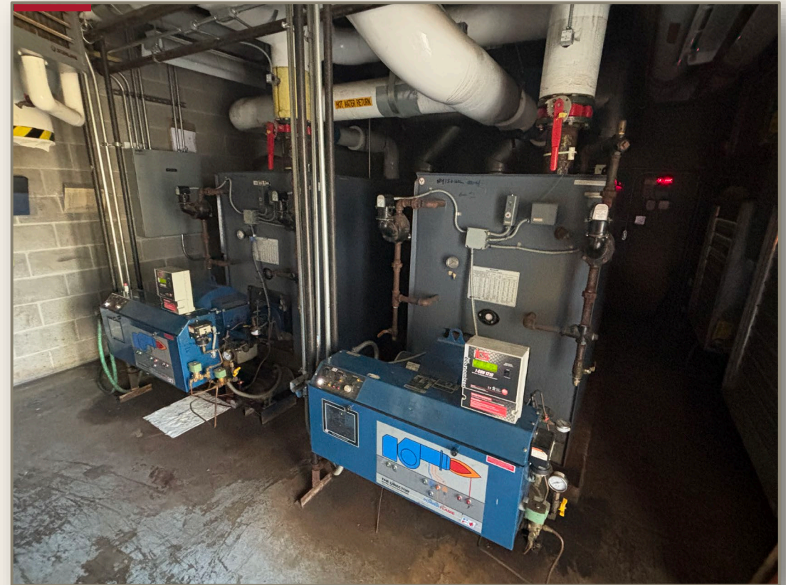
SHS BOILERS TO BE REPLACED
