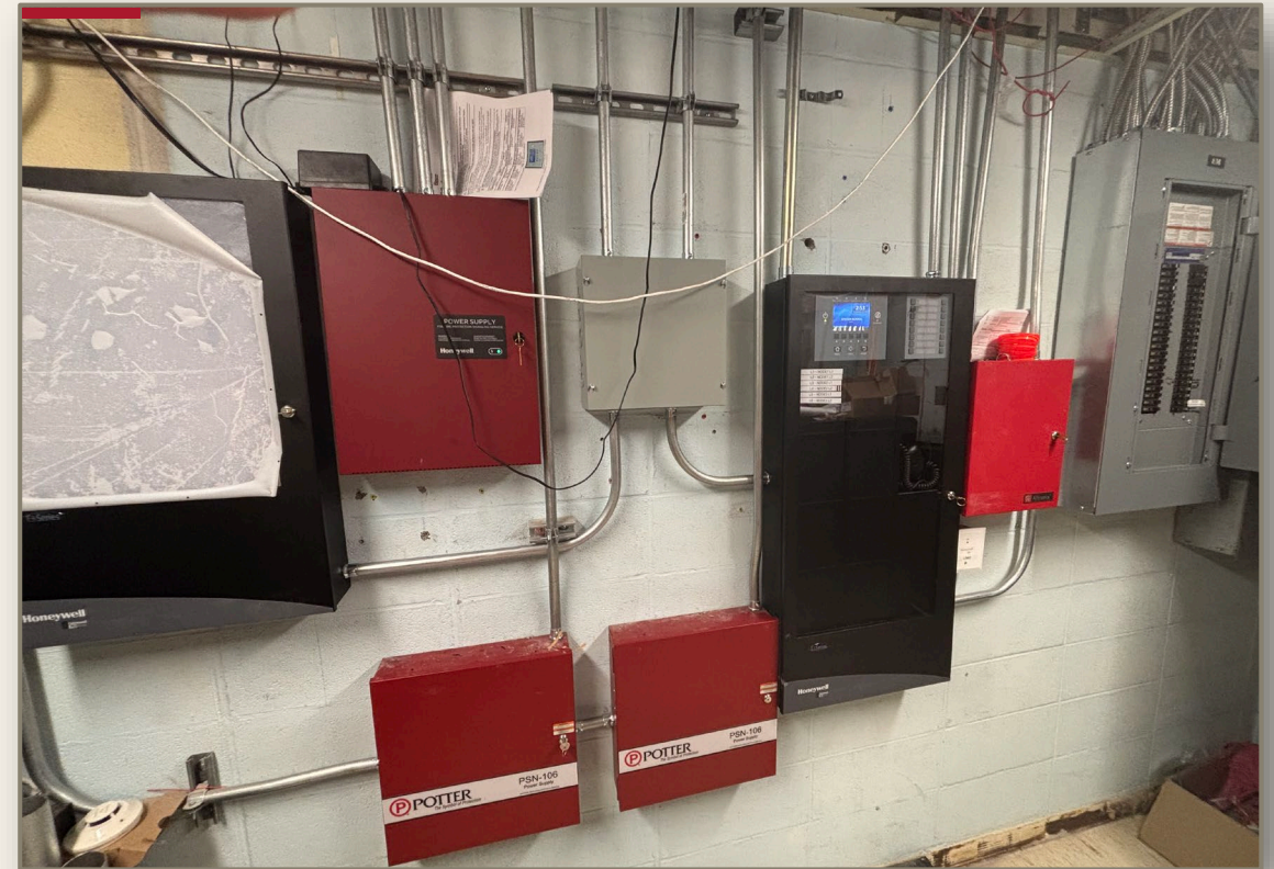
NEW FIRE ALARM PANELS IN SHS
