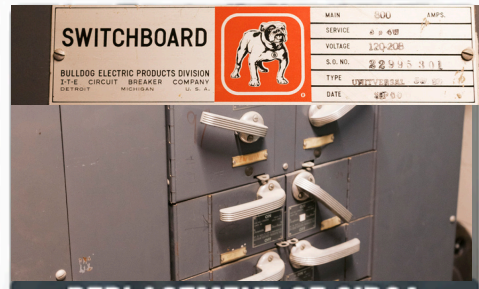
REPLACEMENT OF CIRCA 1960 ELECTRICAL SERVICE
