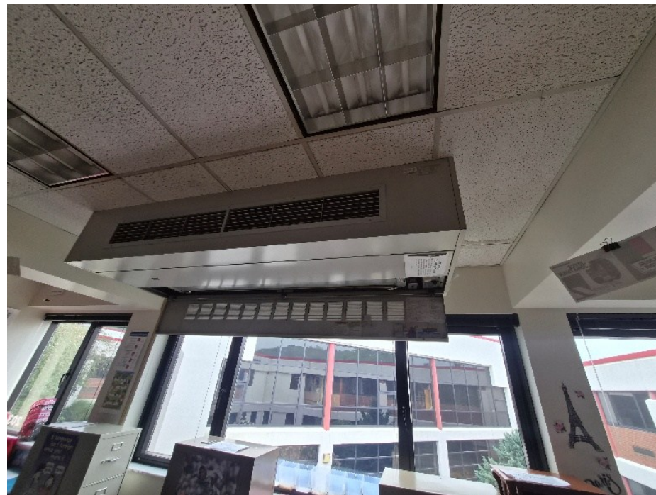
Typical Ceiling Classroom Unit Ventilator
