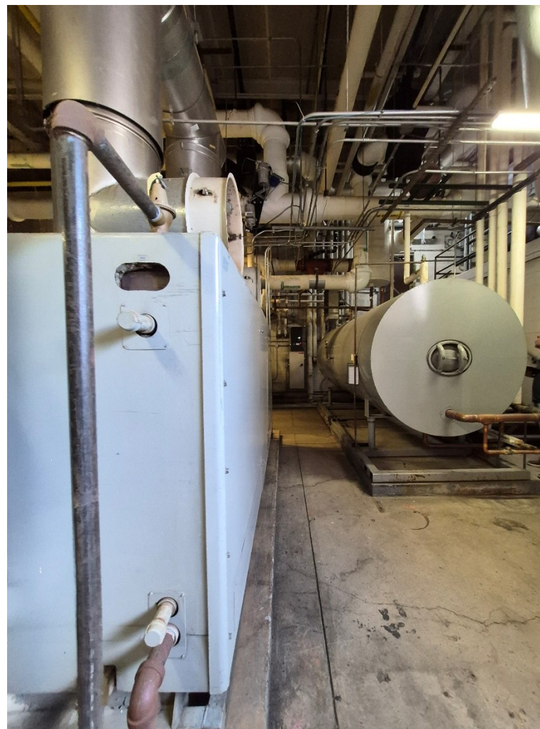
Existing Hot Water Storage Tank
