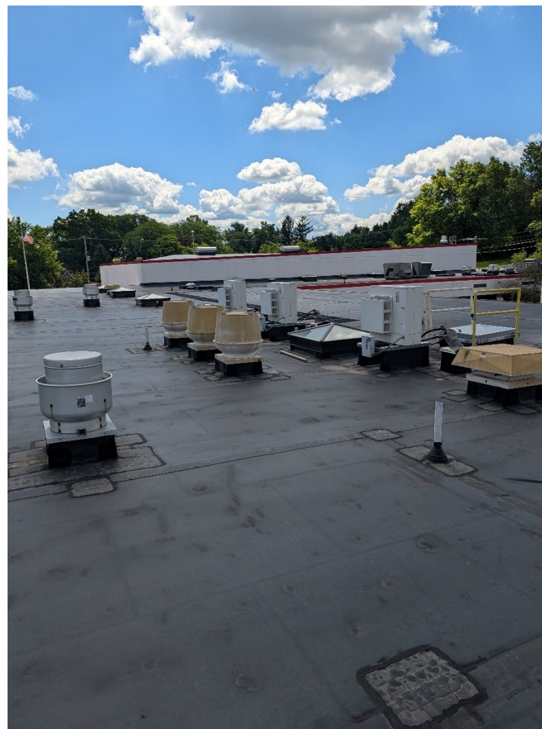
Typical Existing Rooftop Equipment to be Retro-Commissioned
