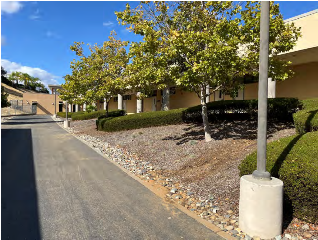
Photo 19 — Minor erosion in a planter near Building E in the western portion of the site.
