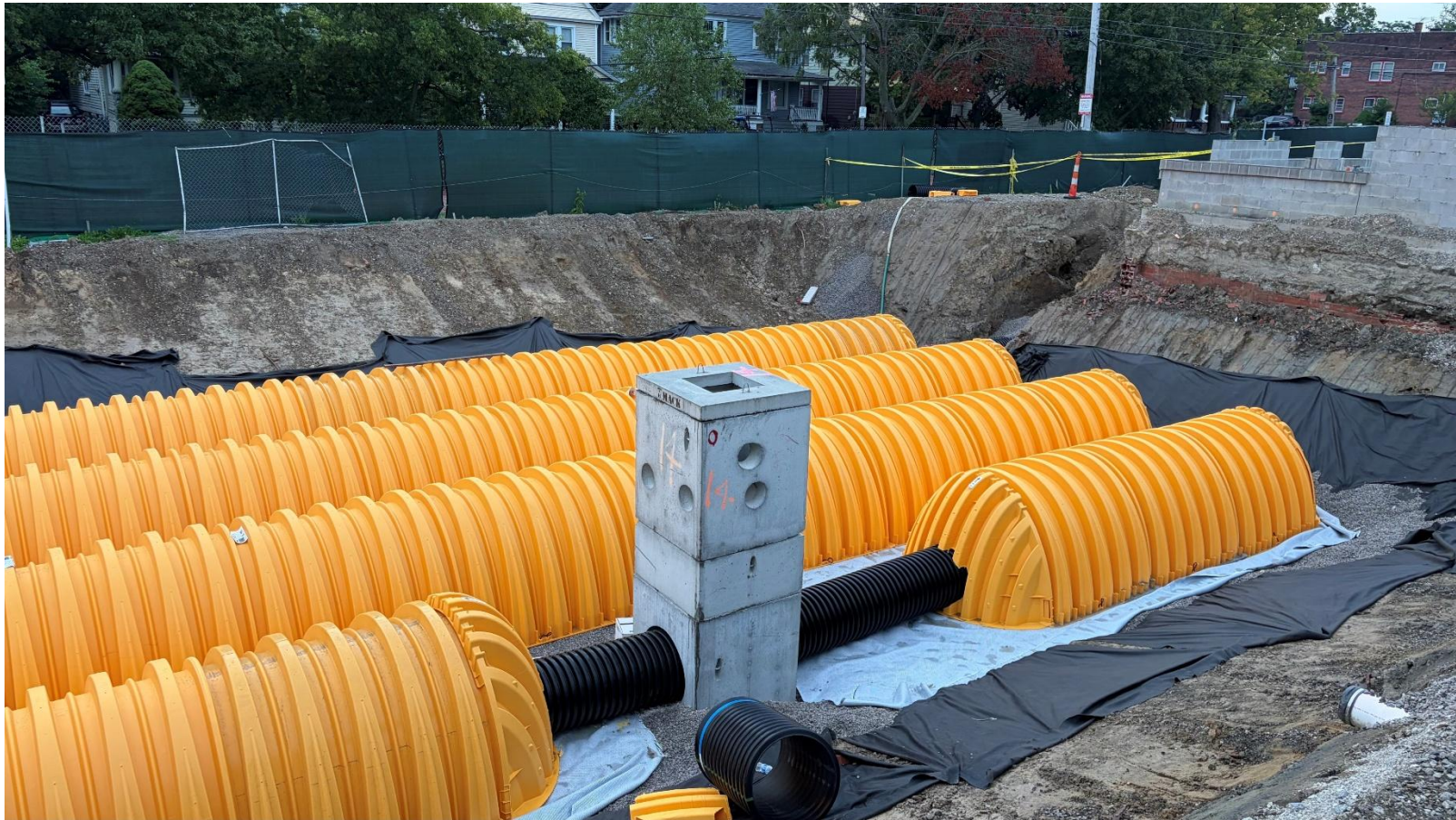
UNDERGROUND RETAINAGE SYSTEM
