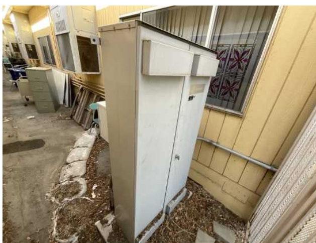
29 - MAIN ELECTRICAL EQUIPMENT
