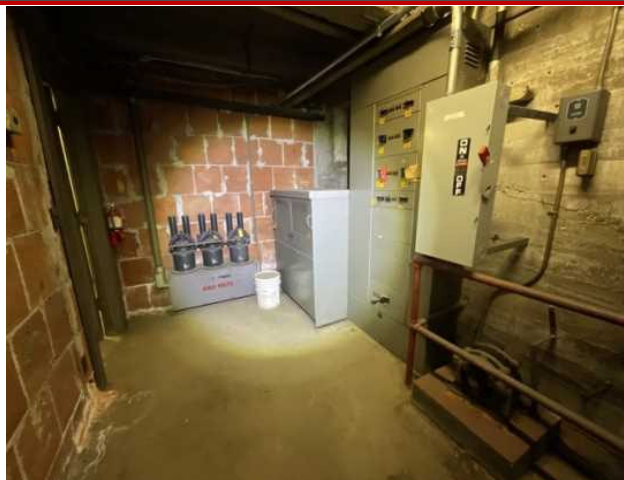
32 - ADMINISTRATION - ELECTRICAL ROOM
