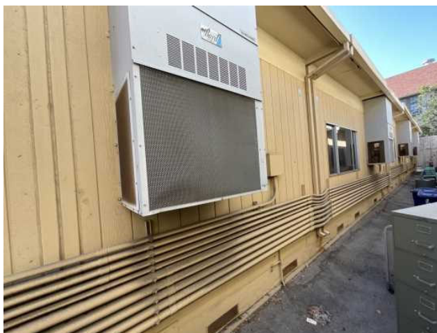
27 - PACKAGED WALL HEAT PUMPS
