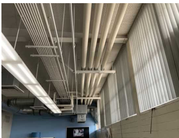
17 - CHILL WATER/STEAM PIPING
