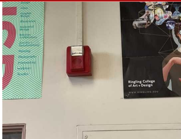
26 - FIRE ALARM STROBE LIGHT
