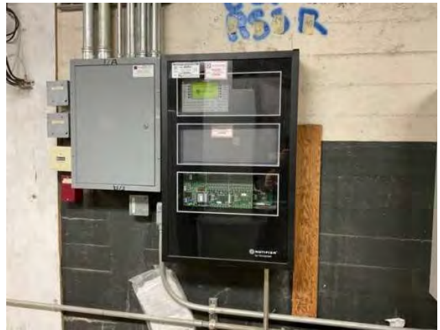
28 - FIRE ALARM PANEL
