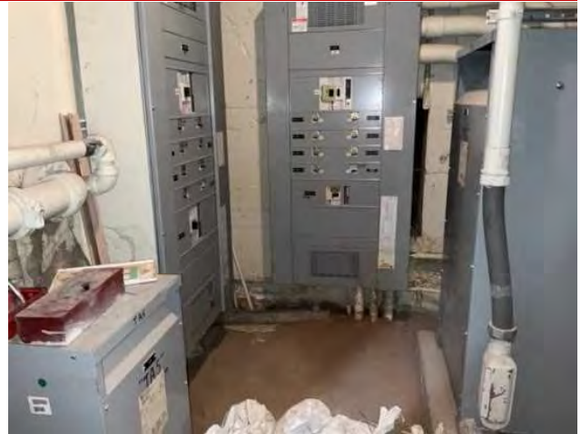
26 - MAIN ELECTRICAL EQUIPMENT
