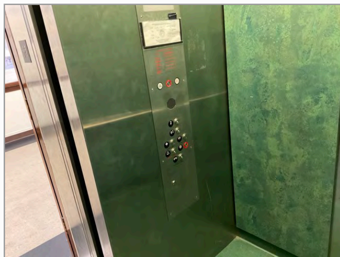
In-cab controls/emergency call panel
