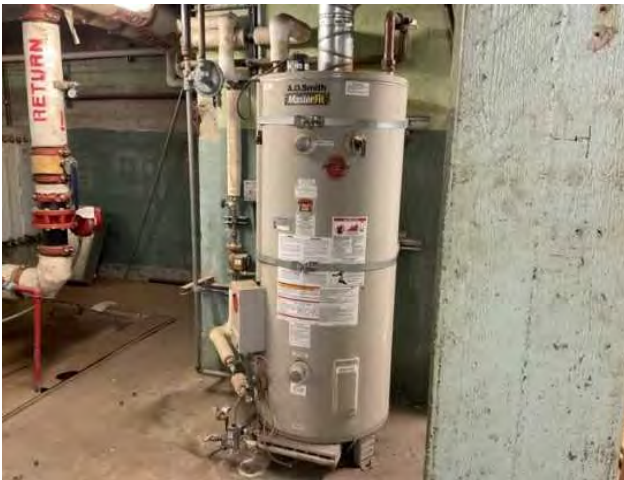
21 - GAS WATER HEATER
