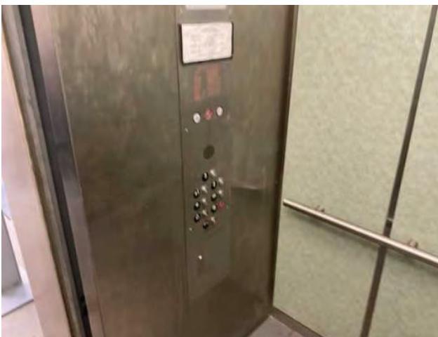
35 - IN-CAB CONTROLS/EMERGENCY CALL PANEL
