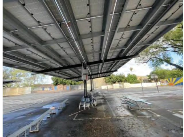
8 - SOLAR POWER SHADED STRUCTURE
