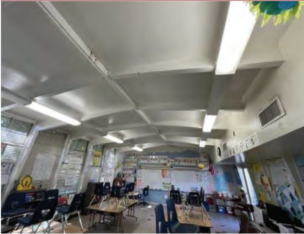
31 - INTERIOR LIGHTING SYSTEM
