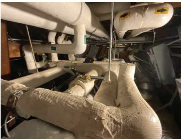
23 - HVAC HYDRONIC PIPING SYSTEM
