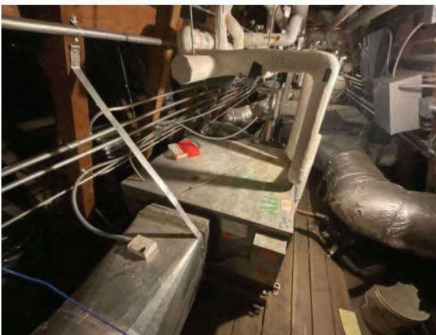
17 - AIR HANDLER AH-18
