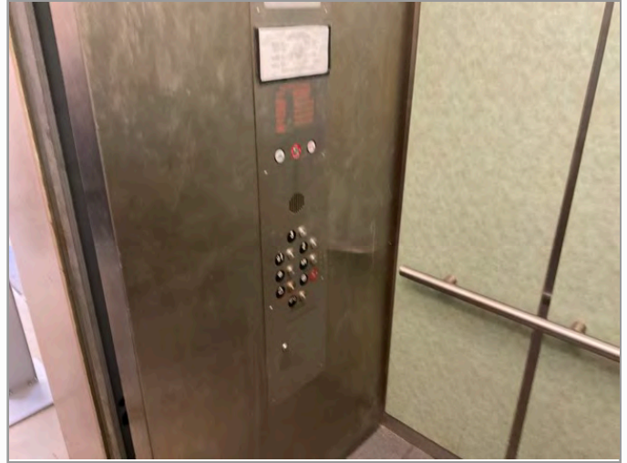
In-cab controls/emergency call panel
