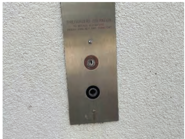
36 - ELEVATOR 1ST FLOOR NO TUMBLER
