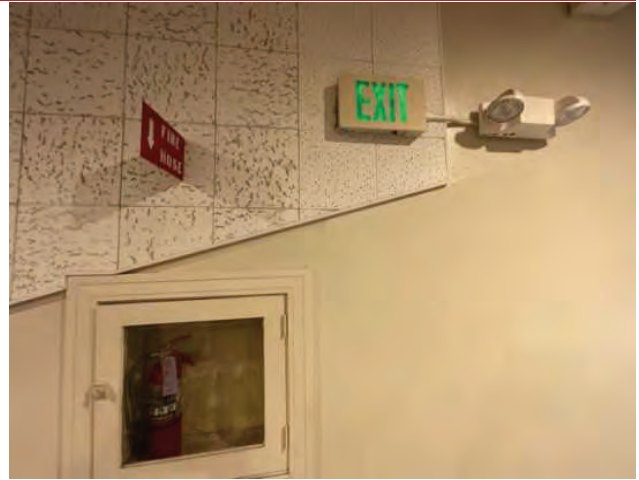
32 - EMERGENCY EXIT AND LIGHTING
