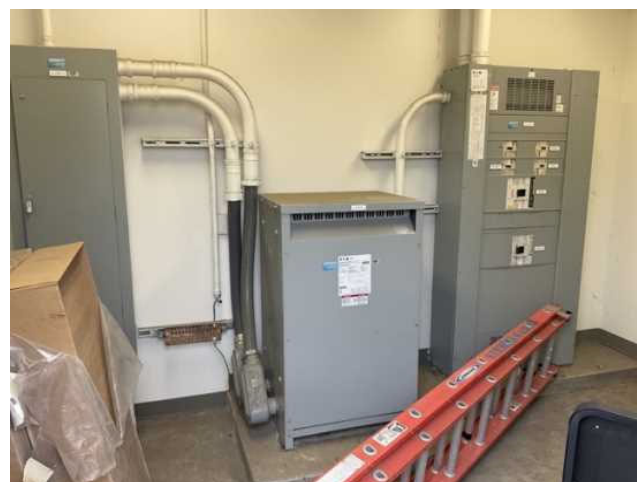
24 - MAIN ELECTRICAL EQUIPMENT
