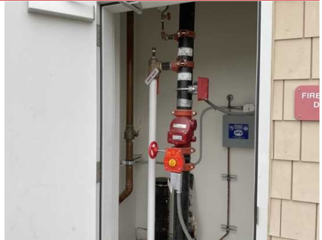
26 - FIRE SUPPRESSION SYSTEM
