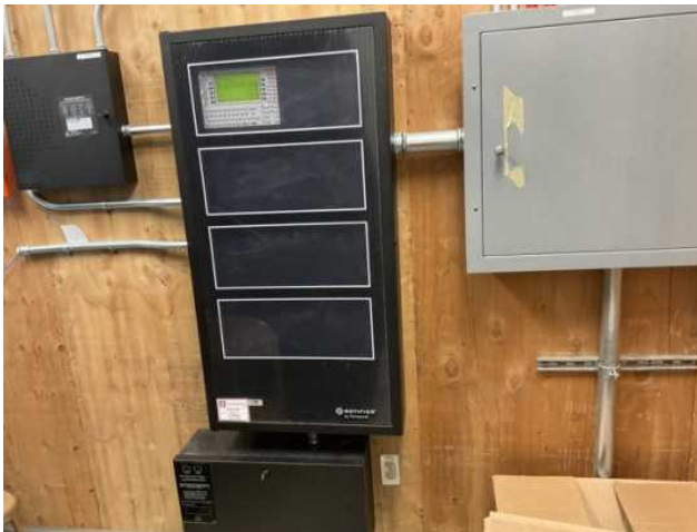
27 - FIRE ALARM PANEL
