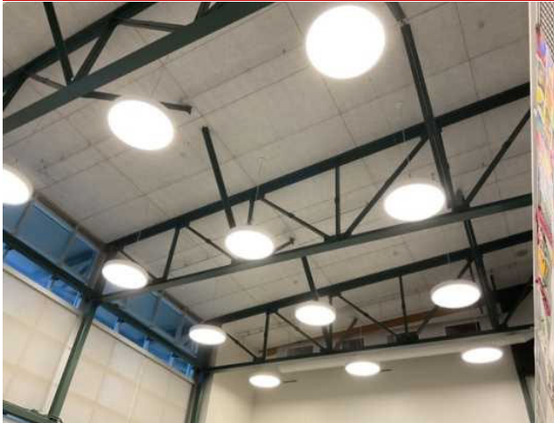
25 - INTERIOR LIGHTING SYSTEM
