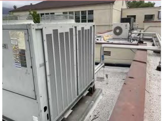
26 - HVAC PACKAGED UNITS
