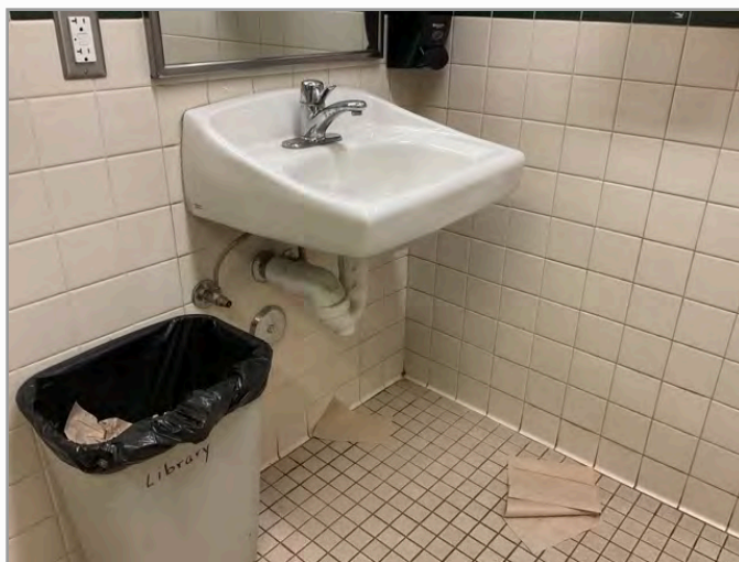
Sink and faucet handles
