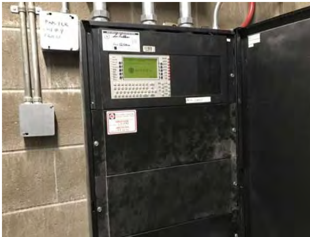
39 - FIRE ALARM PANEL
