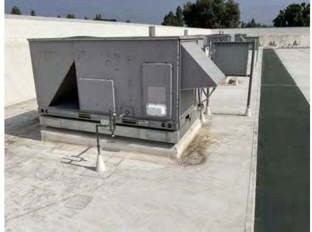
32 – ROOFTOP PACKAGED UNIT
