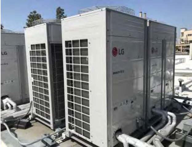
31 - SPLIT SYSTEM DUCTLESS
