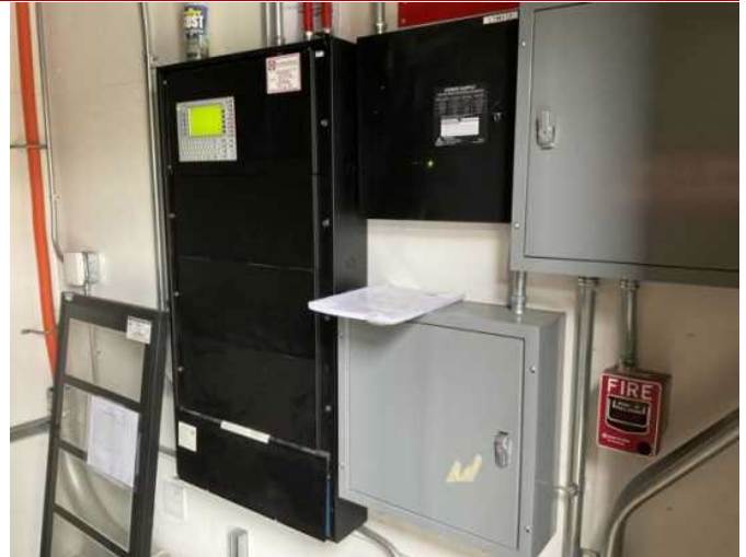
26 - FIRE ALARM PANEL
