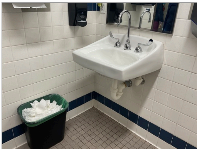
Sink and faucet handles
