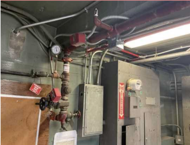
25 - FIRE SUPPRESSION SYSTEM
