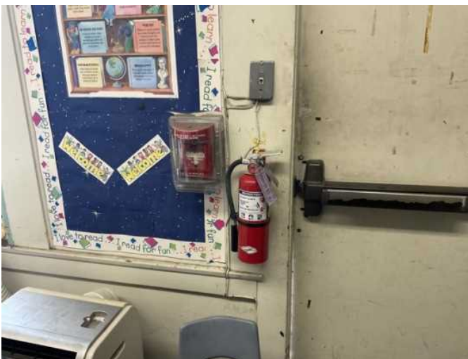
27 - FIRE EXTINGUISHER AND PULL STATION
