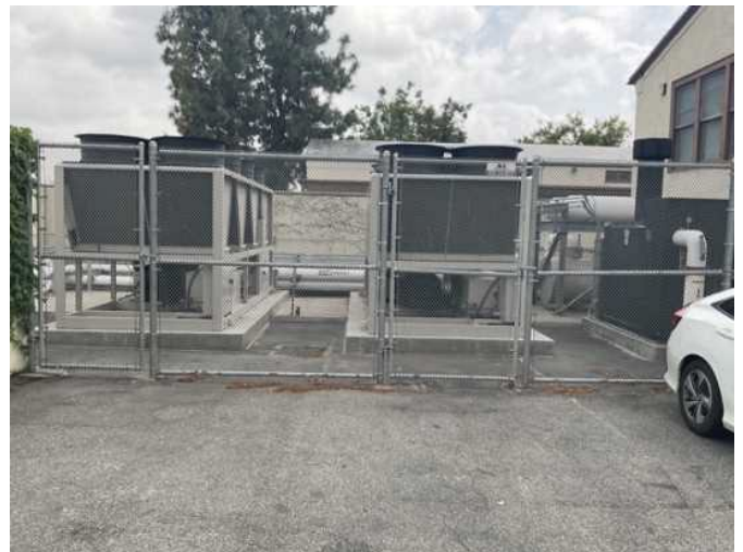
22 - CHILLERS AND BOILER
