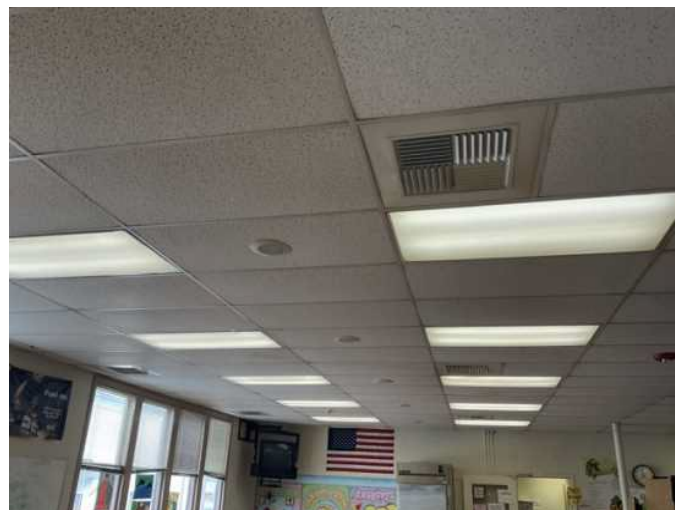
24 - INTERIOR LIGHTING SYSTEM
