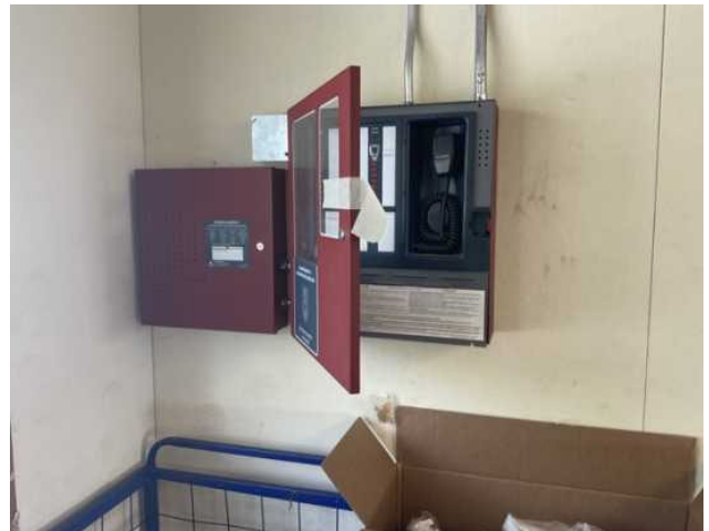
28 - FIRE ALARM PANEL
