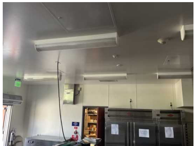
30 - KITCHEN FIRE SUPPRESSION
