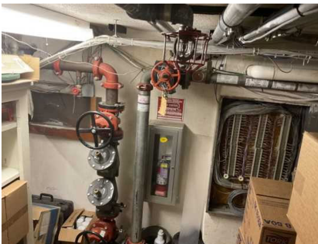
29 - FIRE SUPPRESSION SYSTEM
