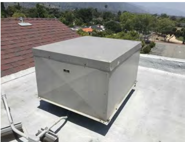
47 - ROOF MOUNTED EXHAUST FAN
