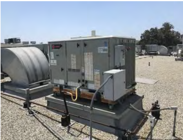
45 - ROOFTOP PACKAGED UNIT (RTU)
