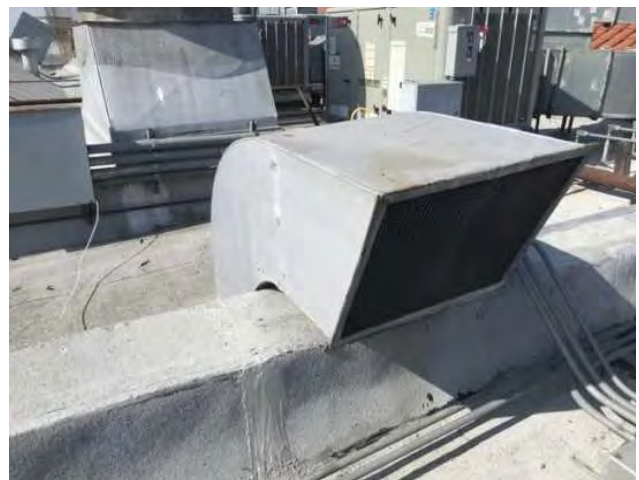
48 - ROOF MOUNTED EXHAUST FAN
