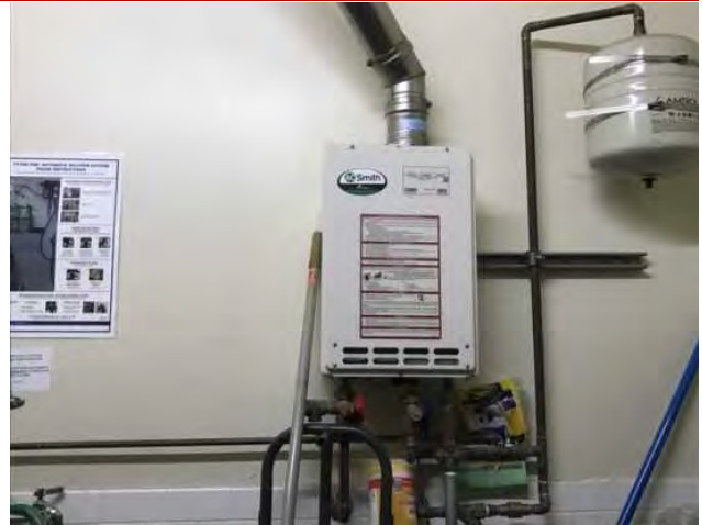
50 – GAS WATER HEATER
