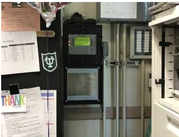
53 - FIRE ALARM PANEL
