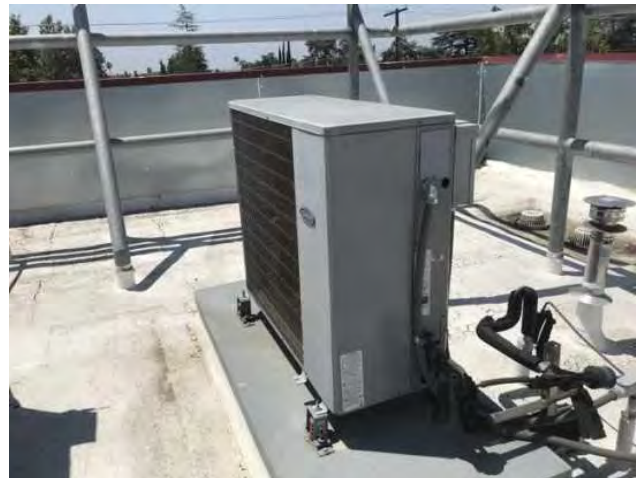
46 - SPLIT SYSTEM CONDENSING UNIT
