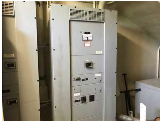
52 – ELECTRICAL DISTRIBUTION PANEL
