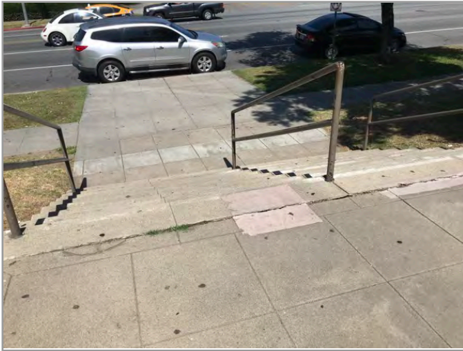
MAIN ENTRANCE IS NOT ACCESSIBLE
