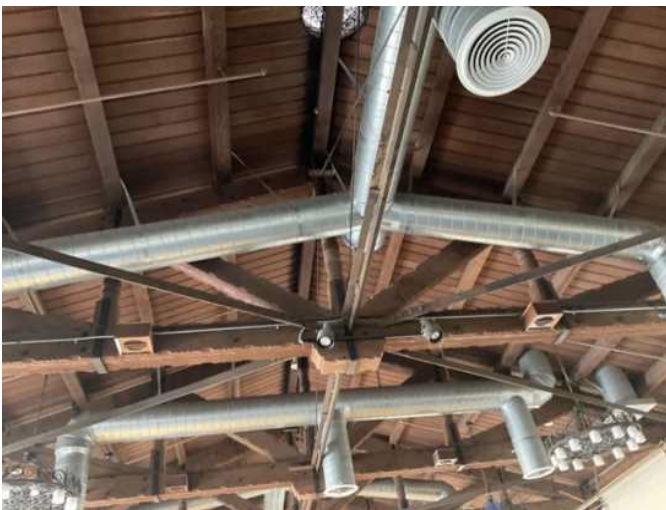
29 - HVAC AIR FLOW INFRASTRUCTURE
