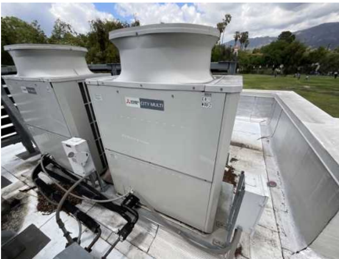
15 - SPLIT SYSTEM BUILDING C
