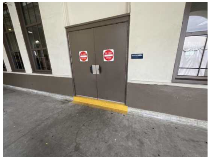
12 - TRIP HAZARD BUILDING B
