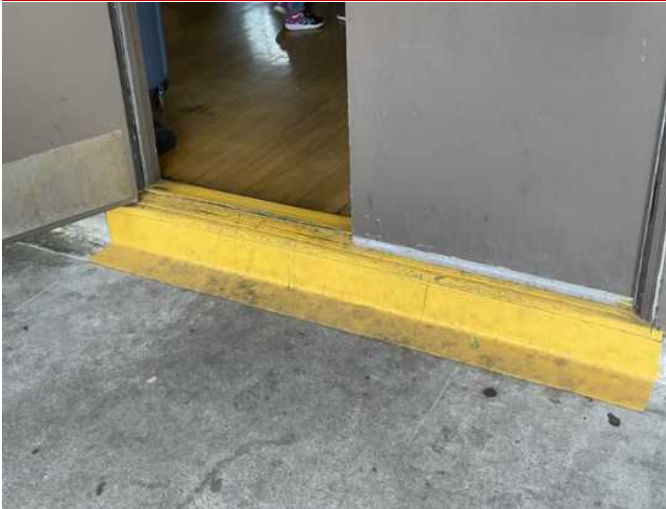
13 - CLOSE-UP TRIP HAZARD BUILDING B
