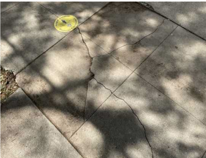
9 - CRACKED CONCRETE PAD ON SOUTH ENTRANCE
