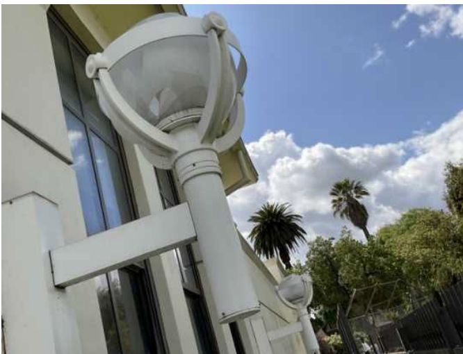
17 - CRACKED EXTERIOR LIGHTS BUILDING C
