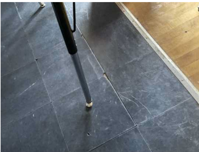
35 - BROKEN/WARPED VCT FLOORING BUILDING A
