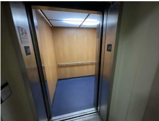
27 - PASSENGER ELEVATOR BUILDING A
