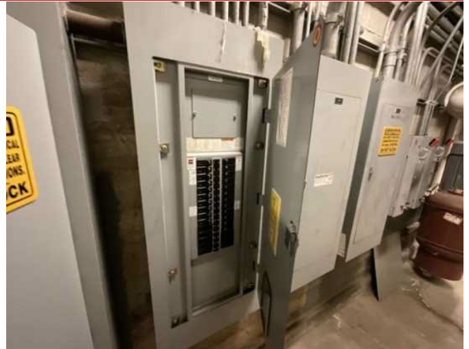
26 - MAIN ELECTRIC DISTRIBUTION ROOM
