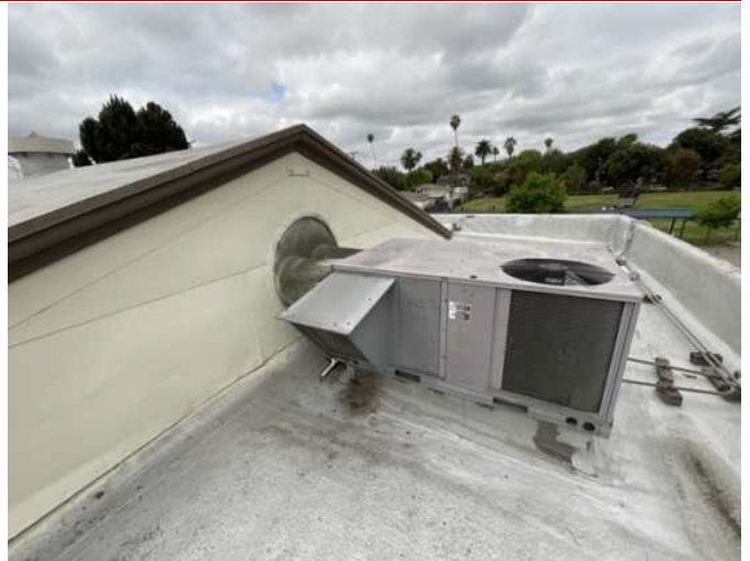
14 - AUDITORIUM RTU BUILDING A
