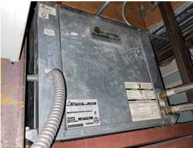
39 - WATER SOURCED HEAT PUMP
