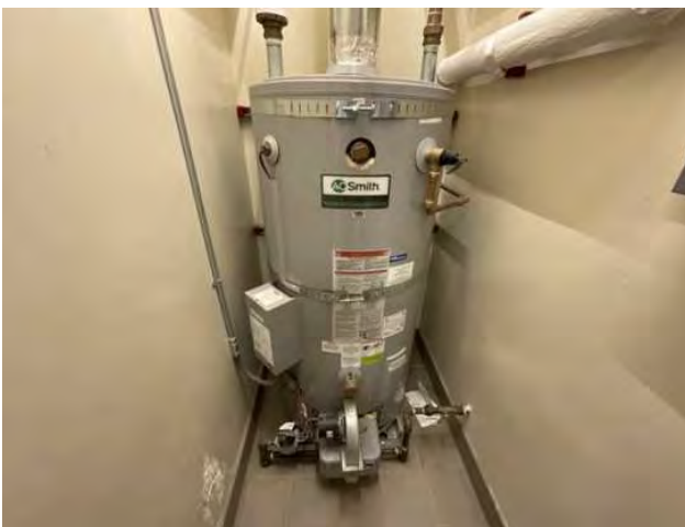
35 - GAS WATER HEATER
