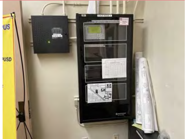
44 - FIRE ALARM PANEL
