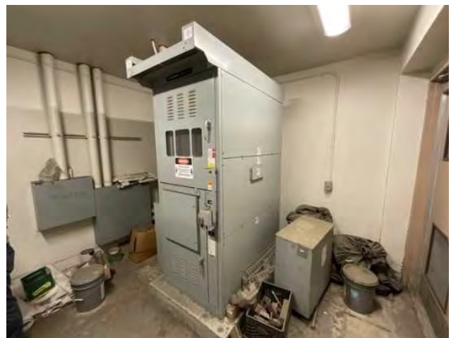
42 - MAIN ELECTRICAL EQUIPMENT
