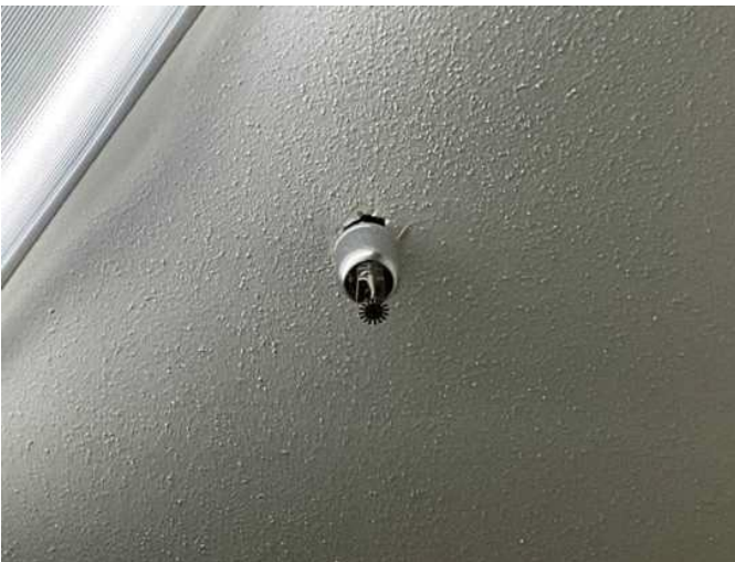
45 - FIRE SUPPRESSION SYSTEM
