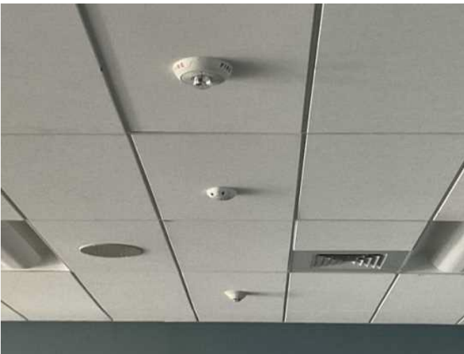
53 - FIRE ALARM SYSTEM
