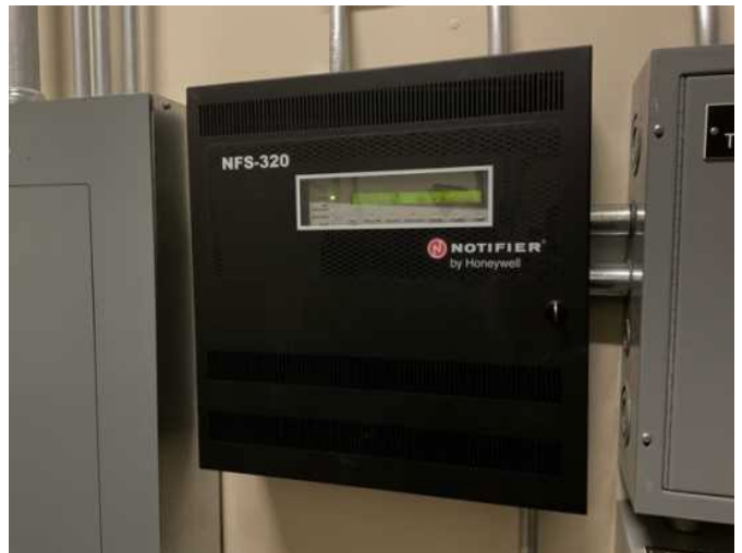
52 - D - FIRE ALARM PANEL
