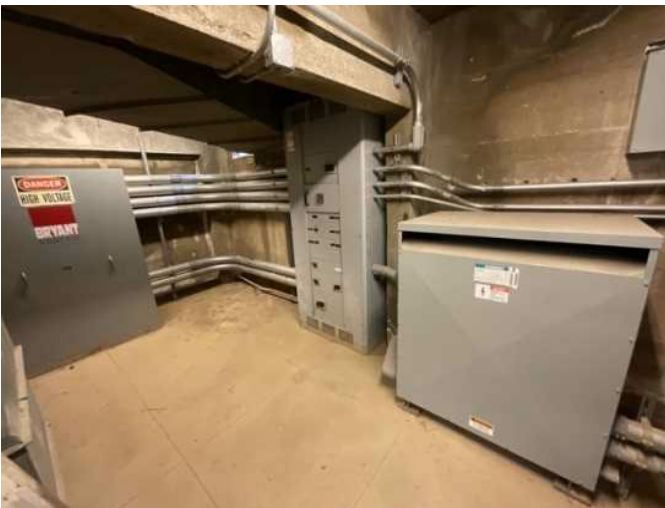
47 - MAIN ELECTRICAL EQUIPMENT
