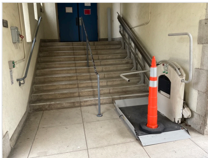
ACCESSIBLE EXTERIOR LIFT
