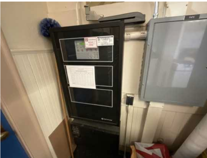
51 - A - FIRE ALARM PANEL
