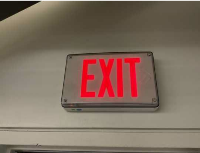
49 - EMERGENCY & EXIT LIGHTING
