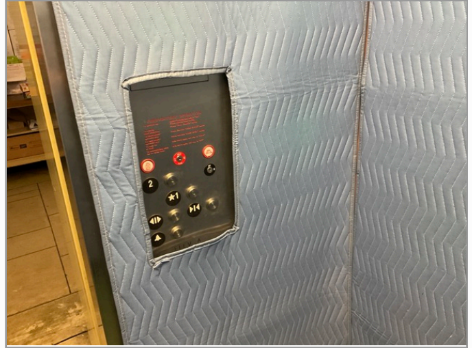
In-cab controls/emergency call panel
