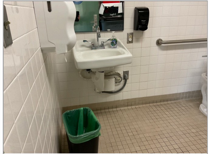
Sink and faucet handles
