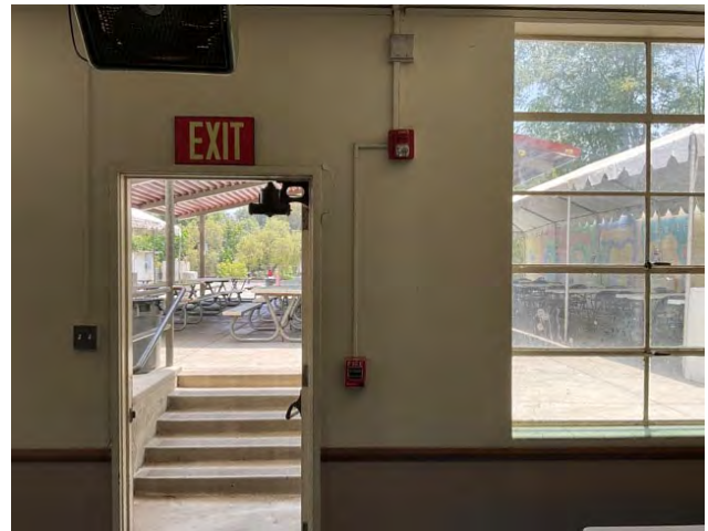
28 - SIGNAGE, STROBE, ALARM, PULL STATION
