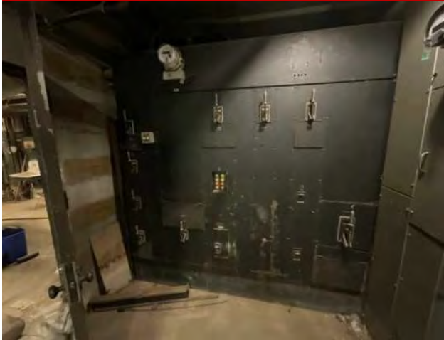
19 - MAIN ELECTRICAL EQUIPMENT
