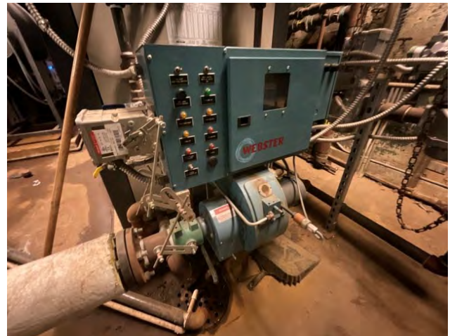
22 - BOILER CONTROL PANEL
