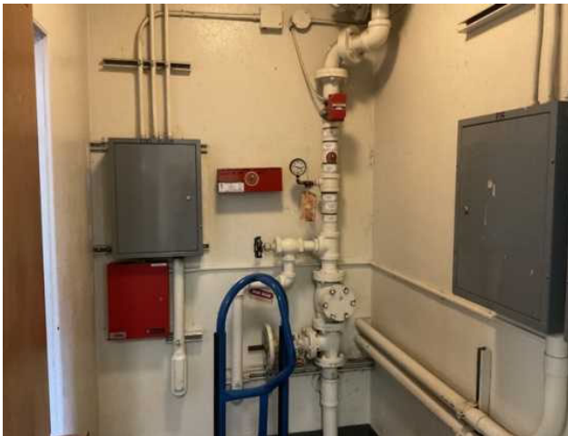
27 - FIRE SUPPRESSION SYSTEM
