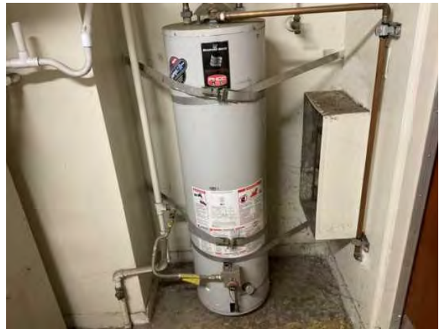
16 - GAS WATER HEATER
