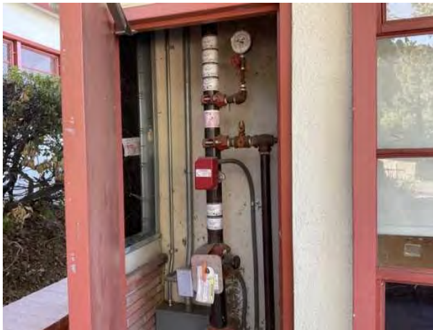
21 - FIRE SUPPRESSION SYSTEM
