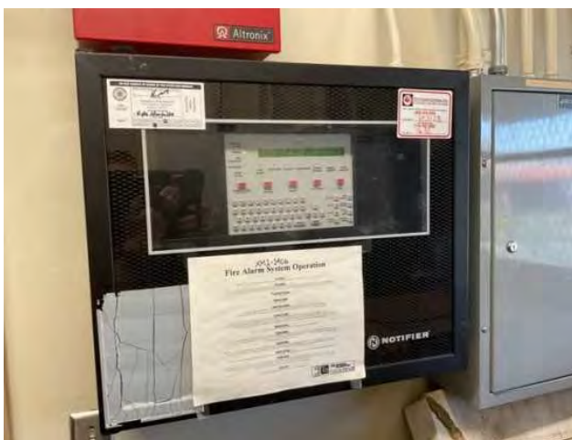
23 - FIRE ALARM PANEL
