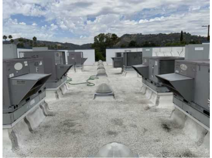
8 - ROOFTOP MECHANICAL EQUIPMENT
