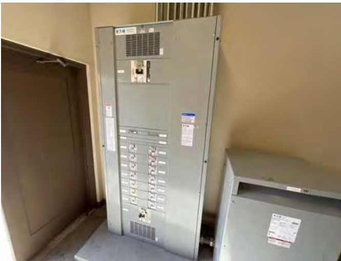
33 - MAIN ELECTRICAL EQUIPMENT
