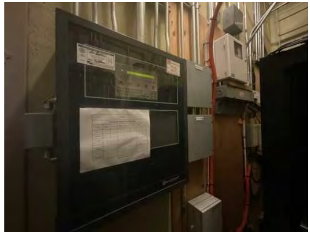
28 - FIRE ALARM PANEL
