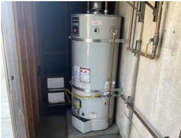
21 - GAS WATER HEATER
