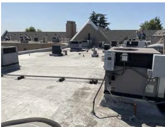
23 - ROOF TOP UNITS
