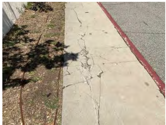
54 - DETERIORATED SIDEWALK, SOUTH SIDE OF A BUILDINGS
