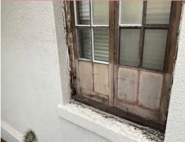
55 - DETERIORATED WOOD WINDOWS, A BUILDING T
