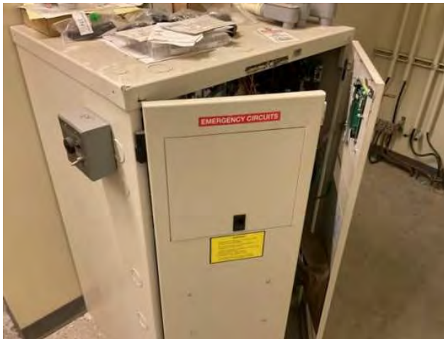
39 - UNINTERRUPTIBLE POWER SUPPLY
