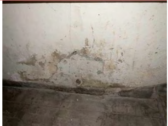
56 - MOISTURE INDUCED DETERIORATION, LOWER LEVEL
