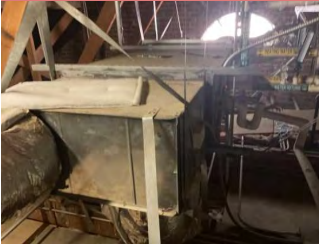
31 - INTERIOR AIR HANDLER
