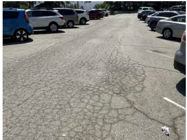
58 - DETERIORATED ASPHALT PAVING
