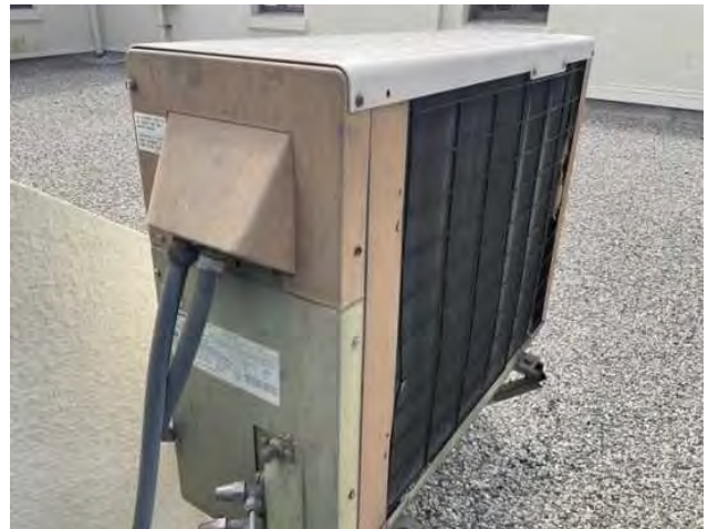
34 - SPLIT SYSTEM DUCTLESS
