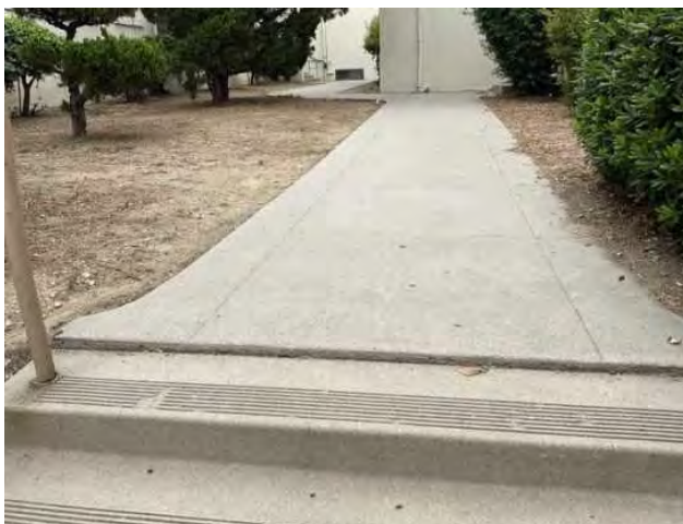
53 - TRIP HAZARD, EAST SIDE BETWEEN A AND C BUILDINGS
