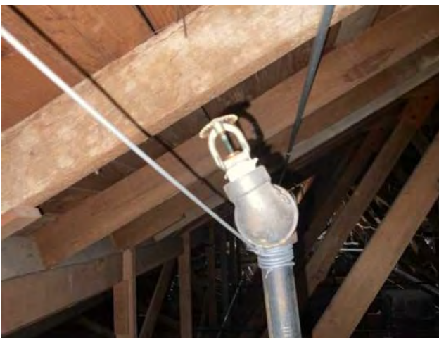
29 - FIRE SPRINKLER SYSTEM
