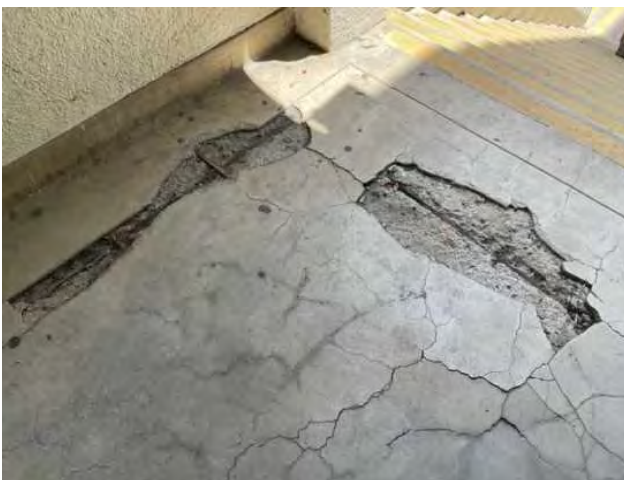
59 - DETERIORATED STEPS EAST SIDE OF A BUILDING
