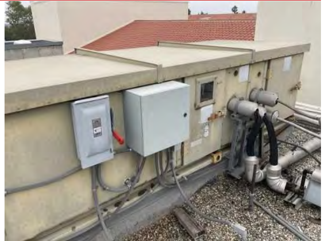
38 - EXTERIOR AIR HANDLER
