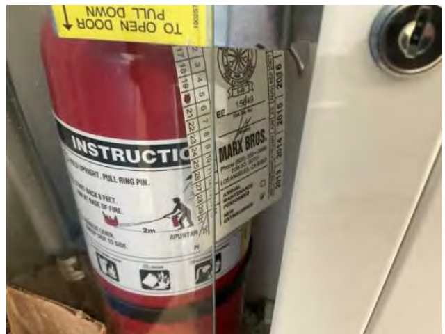
60 - EXPIRED FIRE EXTINGUISHER IN GYMNASIUM
