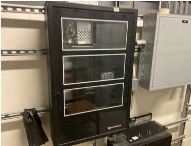
27 - FIRE ALARM PANEL
