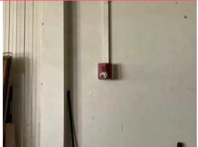
26 - FIRE ALARM SYSTEM
