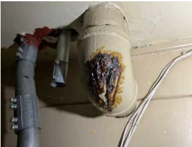
57 - DETERIORATED SANITARY PLUMBING, C BUILDING
