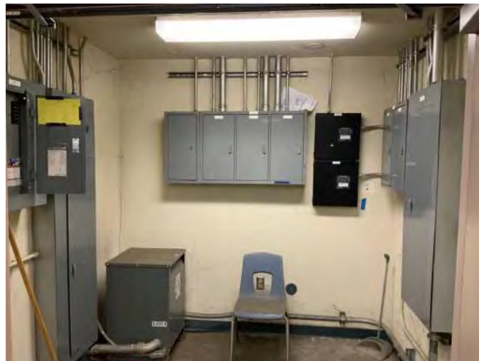
40 - BUILDING B, C, Q, R ELECTRICAL ROOM
