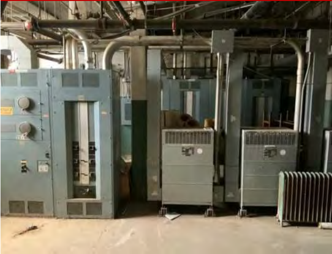
37 - BUILDING A ELECTRICAL ROOM
