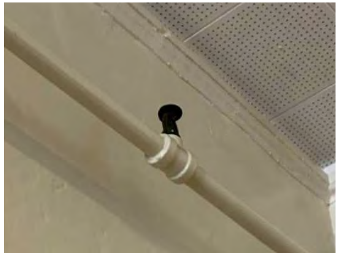
64 - FIRE SUPPRESSION SYSTEM
