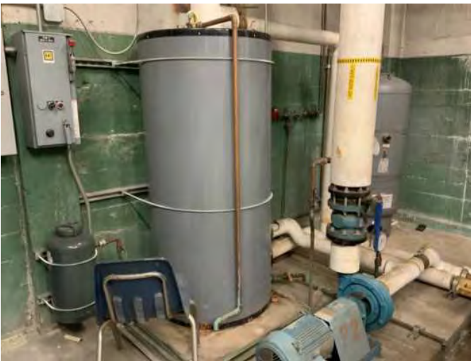
51 - ELECTRIC WATER HEATER
