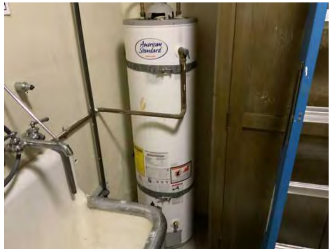
52 - GAS WATER HEATER
