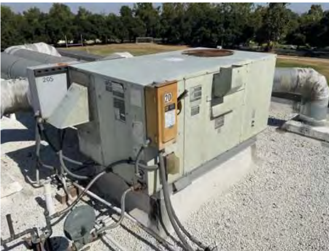
59 - ROOF-TOP PACKAGED UNIT
