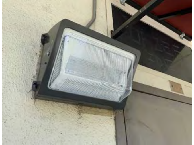
68 - BUILDING MOUNTED LIGHT FIXTURE
