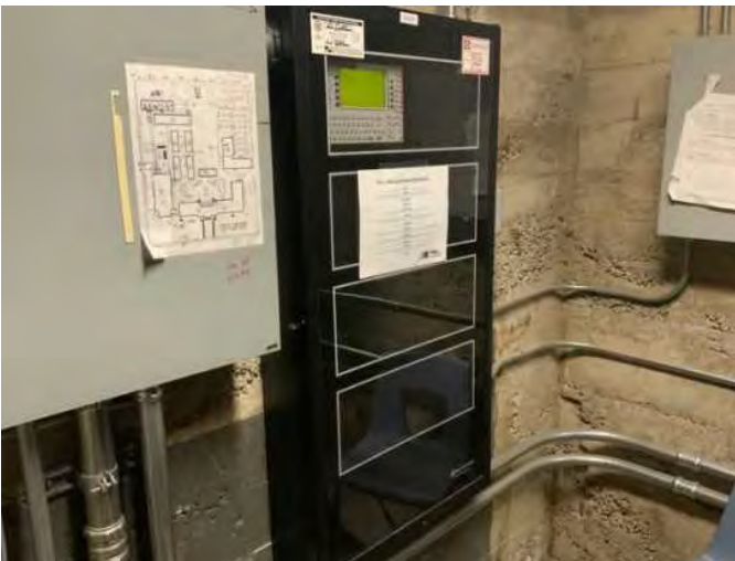
71 - MAIN FIRE ALARM PANEL
