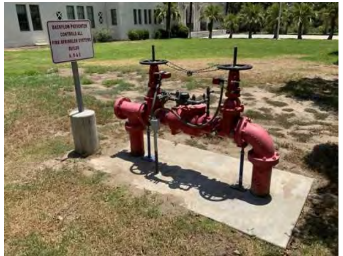
78 - FIRE BACKFLOW PREVENTER
