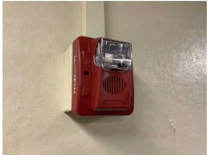
70 - FIRE ALARM SYSTEM
