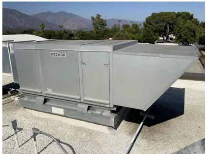
60 - MAKE-UP AIR UNIT
