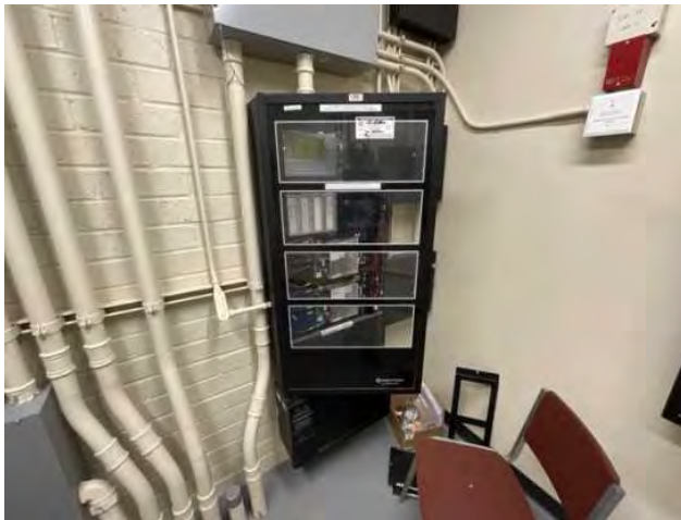
39 - FIRE ALARM PANEL
