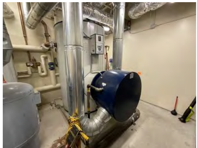
24 - DOMESTIC WATER BOILER
