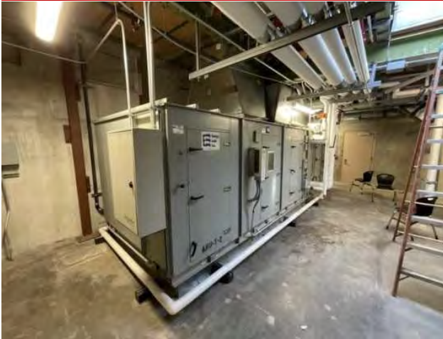
31 - INDOOR AIR HANDLER
