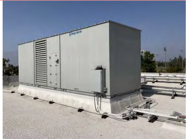
32 - ROOFTOP AIR HANDLER
