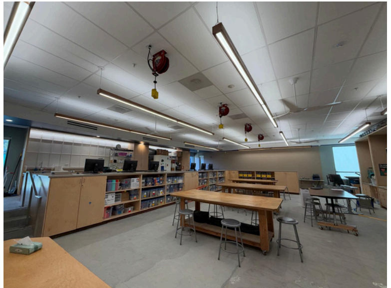
Pictured above : New lighting, new electrical cord reels, and new ceiling fans
