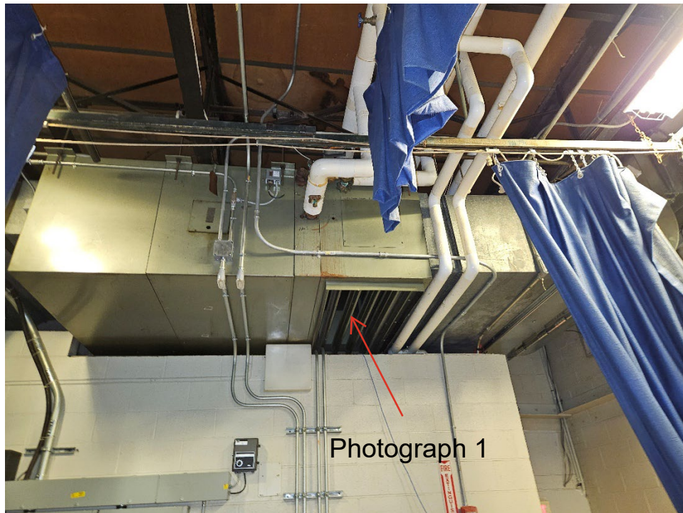
Photograph 2, Stage Air Handler
