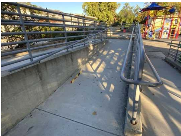
Photos for Barrier ID: AX426463
