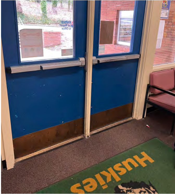
Main entry does not have a secure entry vestibule
