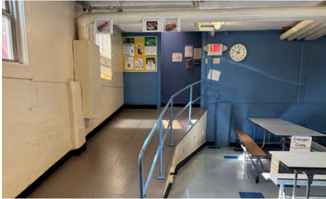
Ramp to enter servery area is not wheelchair accessible
