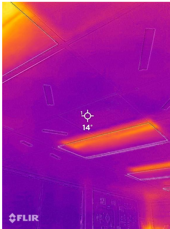
Photo 15. Classroom 131. Thermal image of the ceiling at the supply vent.
