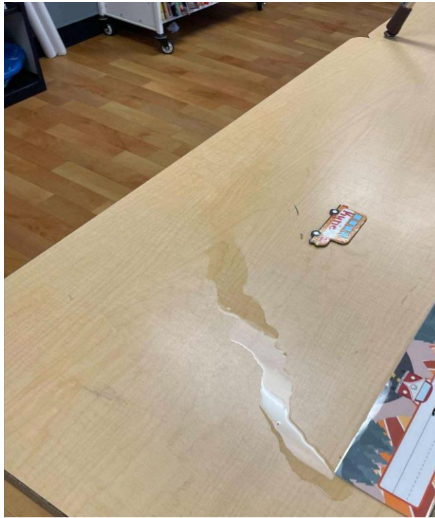
Photo 16. Classroom 131. Standing water on a desktop below the supply vent.
