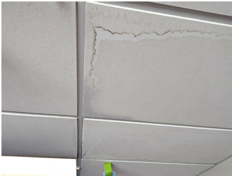
Photo 3. Room 235. Water damage stains on ceiling tiles, second view.
