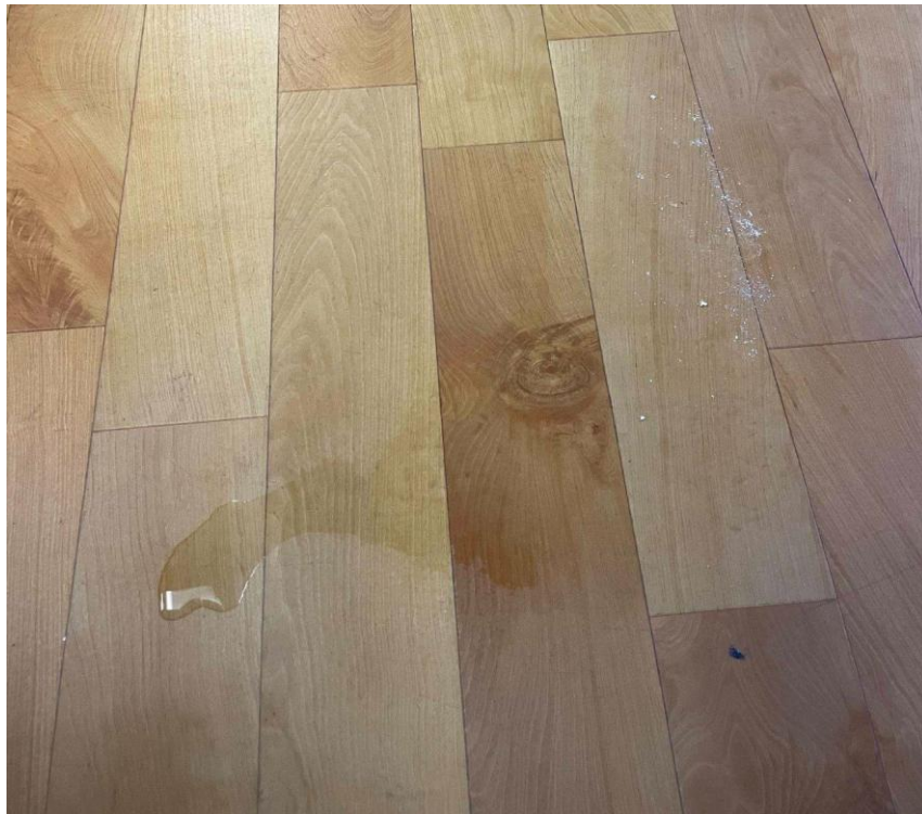
Photo 17. Classroom 131. Water on the floor, suspected to have originated from the supply vent above.
