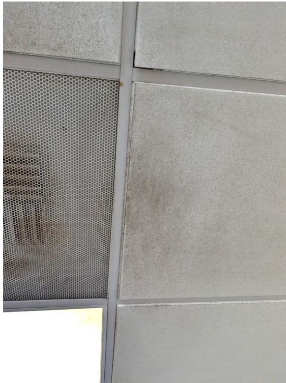
Photo 1. Room 235. Suspect mold staining on the supply vent and adjacent ceiling tile.
