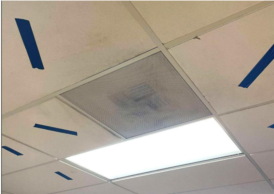
Photo 14. Classroom 131. Supply vent and surrounding ceiling tiles above the area where water was observed.
