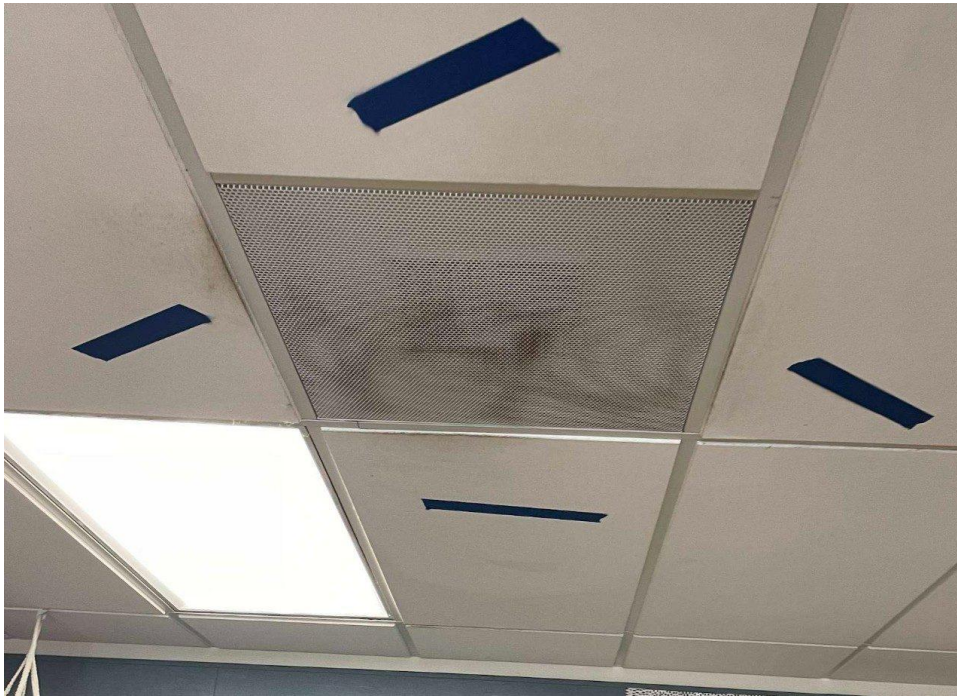
Photo 18. Classroom 118. Suspect mold staining on ceiling tiles adjacent to the supply vent.
