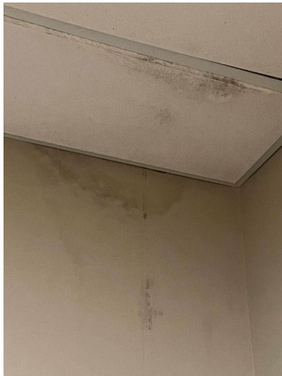
Photo 11. Studio 134. Water damage and mold growth at the ceiling and the wall shared with the mechanical/storage room.
