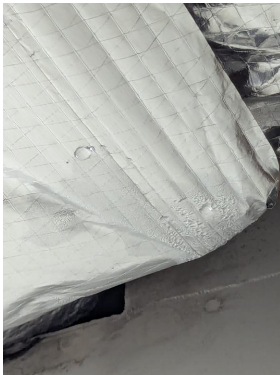
Photo 9. Mechanical/storage room. Condensation droplets on the duct insulation jacket.
