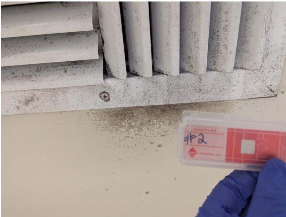
Photo 5. Boys' bathroom, second floor. Surface sample 2 collection location; suspect mold on the vent grille and adjacent ceiling.
