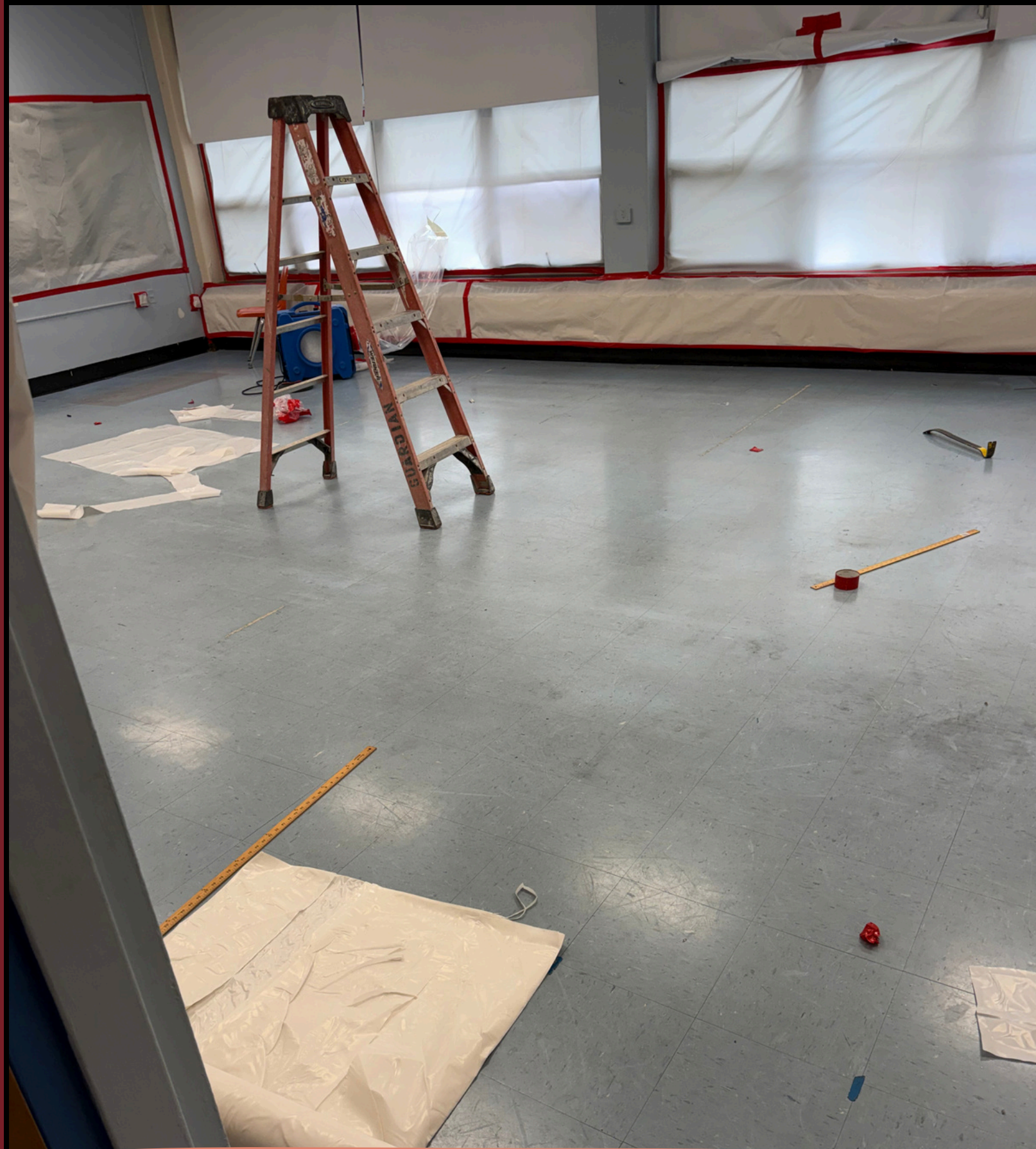
Sussex Avenue Classroom Floors - Before
