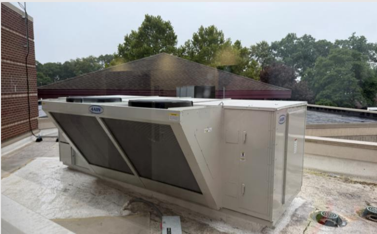
Pembroke – HVAC Unit
