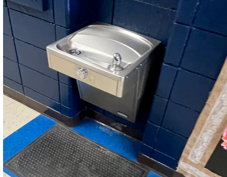
Building Systems - Drinking Fountains
