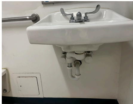
Building Systems - Plumbing Fixtures (Restrooms)
