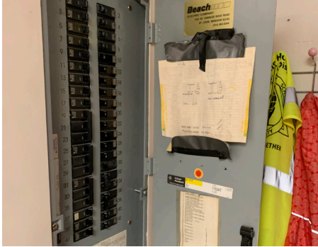
Building Systems - Panelboards
