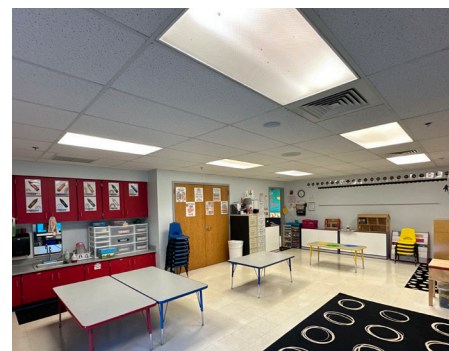
Building Systems - Interior Lighting (Classrooms)
