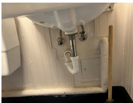
Building Systems - Plumbing (Restrooms)
