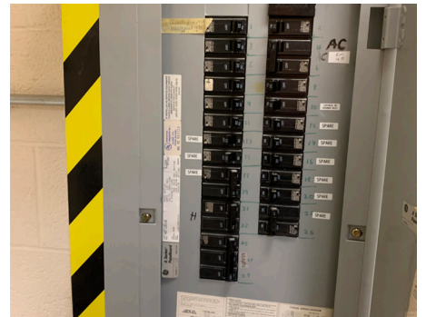
Building Systems - Panelboards
