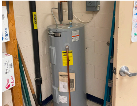
Building Systems - Water Heaters
