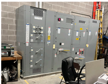
Building Systems - Main Electrical System
