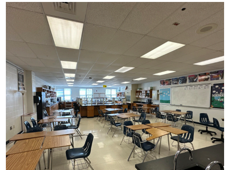
Building Systems - Interior Lighting (Classrooms)
