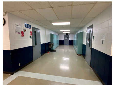
Building Systems - Interior Lighting (Public Areas)
