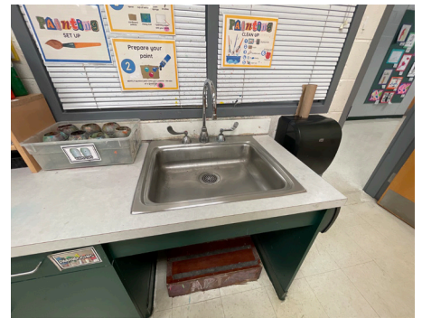
Building Systems - Plumbing Fixtures (Classroom)
