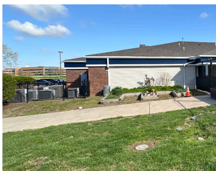
Building Systems - Mechanical System
