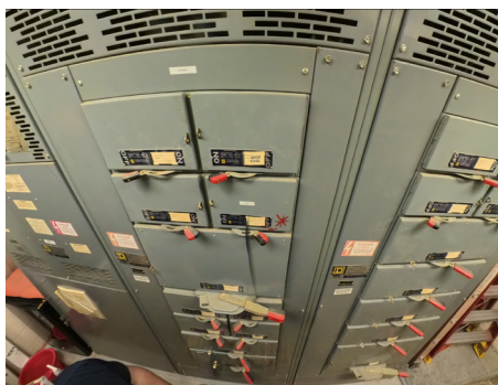
Building Systems - Main Electrical Service
