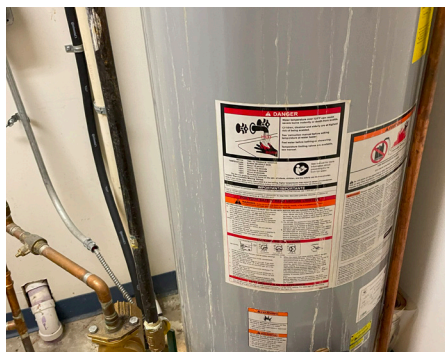
Building Systems - Water Heaters
