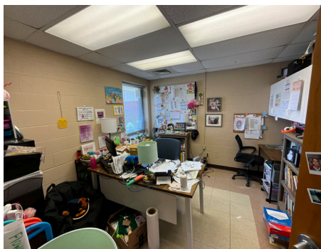
Building Systems - Interior Lighting (Classrooms)
