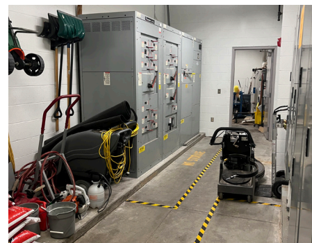
Building Systems - Main Electrical Service
