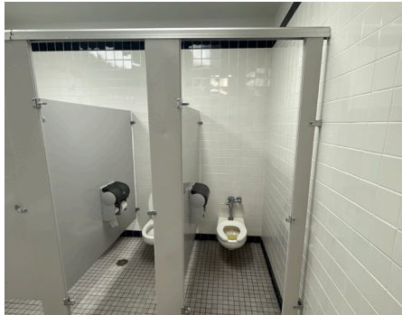
Building Systems - Plumbing Fixtures (Restrooms)
