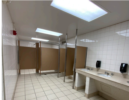
Building Systems - Plumbing Fixtures (Restrooms)
