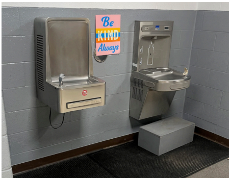
Building Systems - Drinking Fountains
