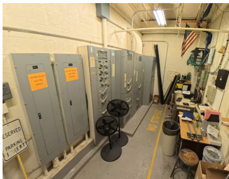
Building Systems - Main Electrical Service
