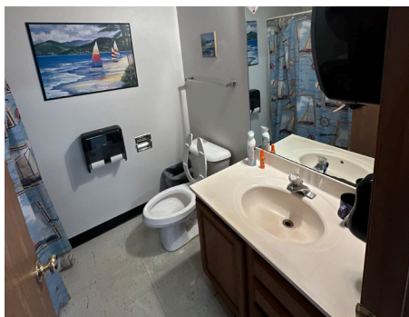
Building Systems - Plumbing Fixtures (Restrooms)
