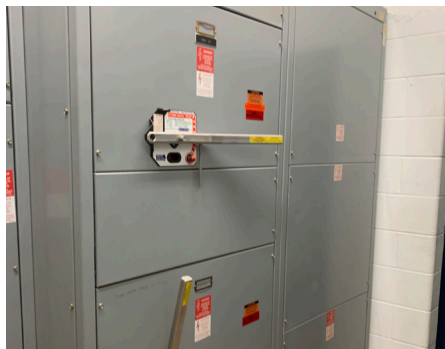
Building Systems - Main Electrical Service
