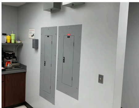
Building Systems - Panelboards
