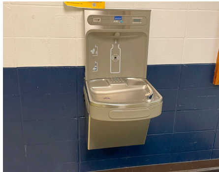
Building Systems - Drinking Fountains
