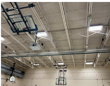
Building Systems - Interior Lighting (Public Areas)
