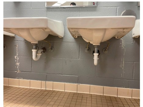
Building Systems - Plumbing Fixtures (Restrooms)
