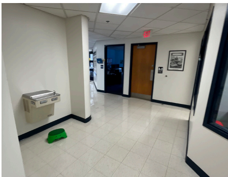
Building Systems - Drinking Fountains
