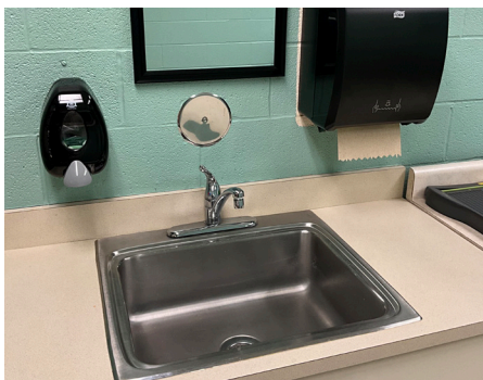
Building Systems - Plumbing Fixtures (Classrooms)
