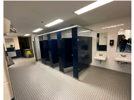
Interior Environment - Plumbing Fixture
