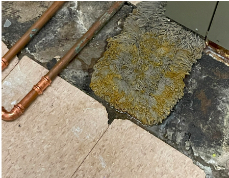
Building Systems - Mechanical System
