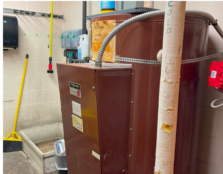
Building Systems - Water Heaters
