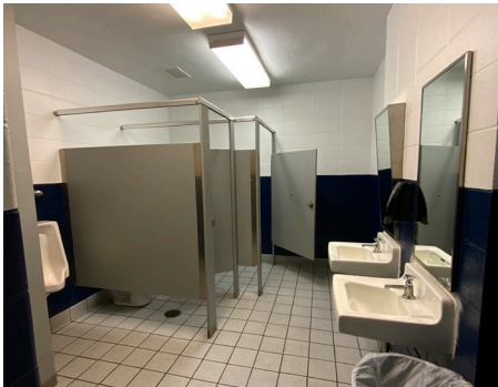
Building Systems - Plumbing Fixtures (Restrooms)
