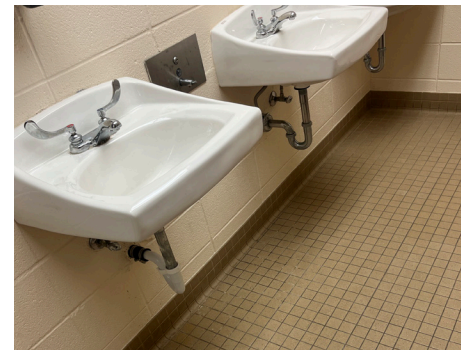
Building Systems - Plumbing Fixtures (Restroom)
