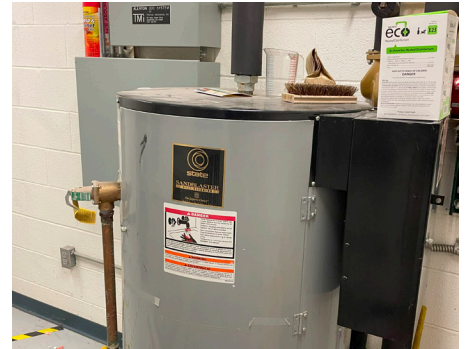
Building Systems - Water Heaters
