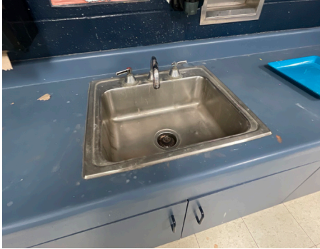
Building Systems - Plumbing Fixtures (Classrooms)
