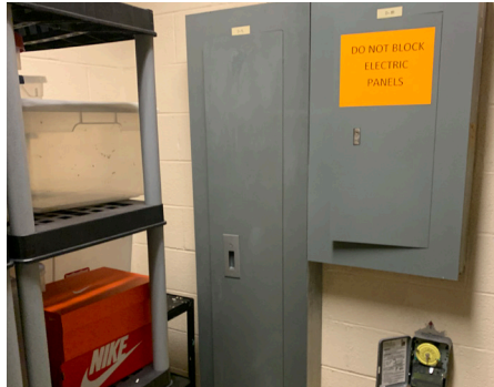
Building Systems - Panelboards
