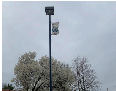
Building Site - Site Lighting
