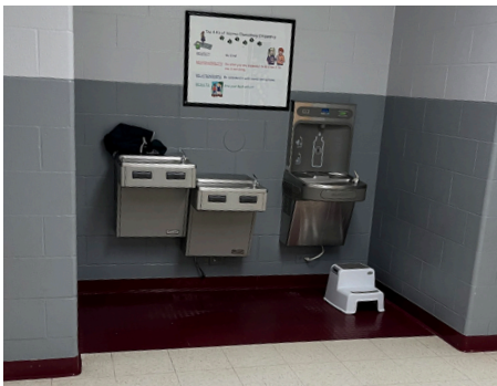
Building Systems - Drinking Fountains
