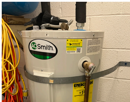
Building Systems - Water Heaters
