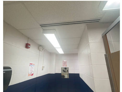
Building Systems - Interior Lighting (Public Areas)
