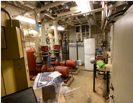
Building Systems - Water Heaters
