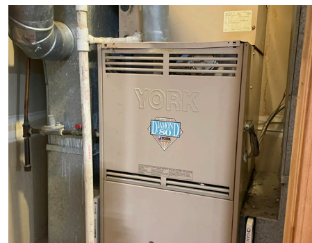
Building Systems - Mechanical Systems
