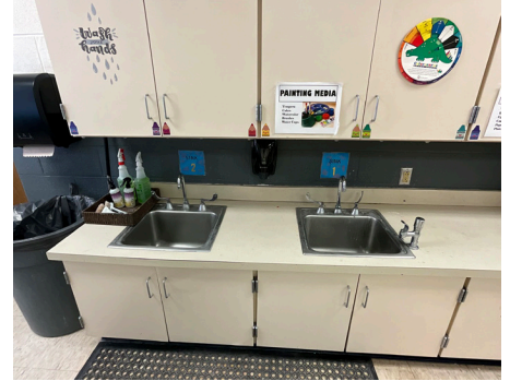
Building Systems - Plumbing Fixtures (Classroom)
