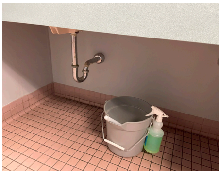
Building Systems - Plumbing Fixtures (Restrooms)
