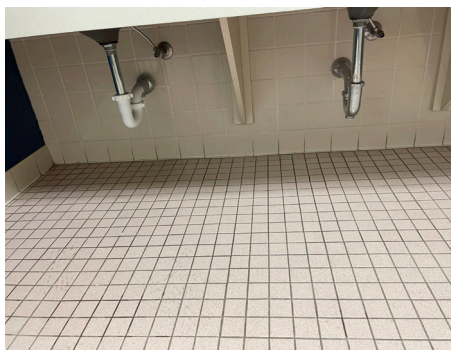
Building Systems - Plumbing Fixtures (Restrooms)
