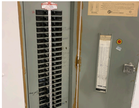
Building Systems - Panelboards
