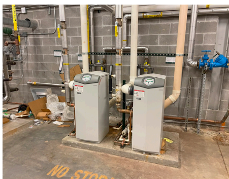
Building Systems - Water Heaters
