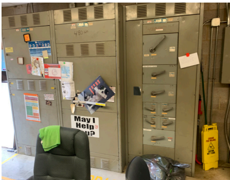
Building Systems - Main Electrical Service
