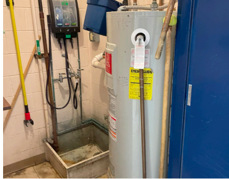
Building Systems - Water Heaters
