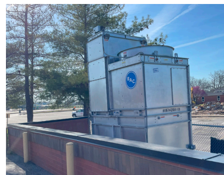
Building Systems - Mechanical System
