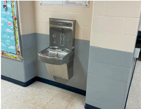
Building Systems - Drinking Fountains
