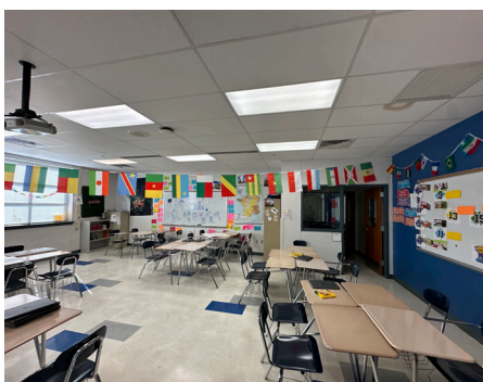
Building Systems - Interior Lighting (Classrooms)
