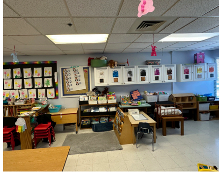
Building Systems - Interior Lighting (Classrooms)
