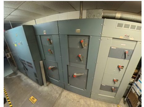
Building Systems - Main Electrical System
