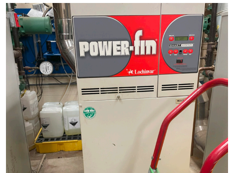
Building Systems - Mechanical System
