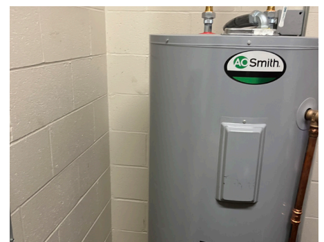
Building Systems - Water Heaters
