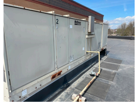
Building Systems - Mechanical System
