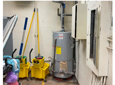
Building Systems - Water Heaters
