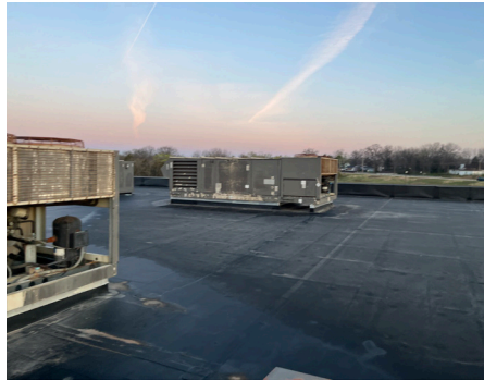
Building Systems - Mechanical System
