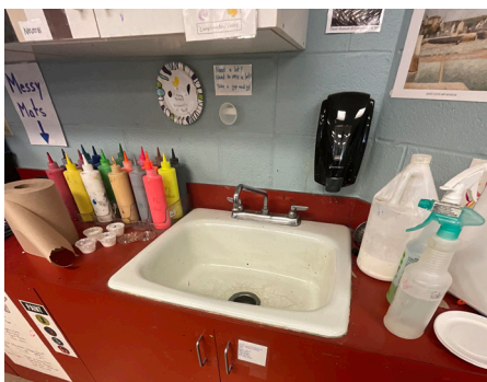
Interior Environment - Casework
