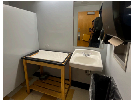
Building Systems - Plumbing Fixtures (Restrooms)
