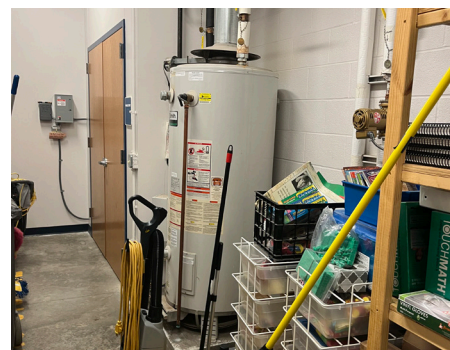
Building Systems - Water Heaters
