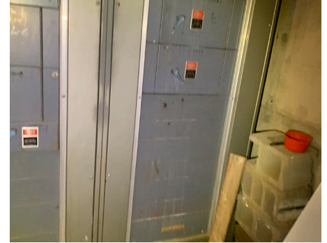
Building Systems - Main Electrical Systems
