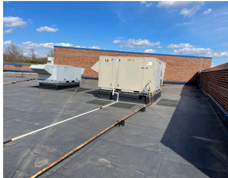
Building Systems - Mechanical System
