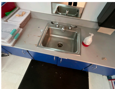
Building Systems - Plumbing Fixtures (Classrooms)
