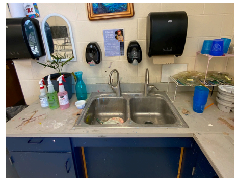
Building Systems - Plumbing Fixtures (Classroom)
