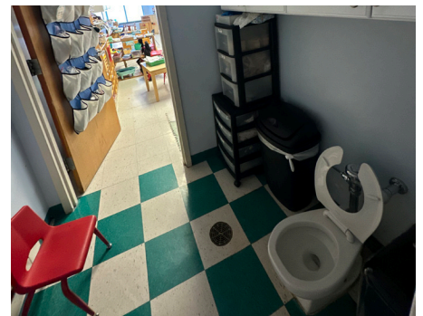
Building Systems - Plumbing Fixtures (Classrooms)
