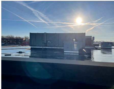
Building Systems - Mechanical System
