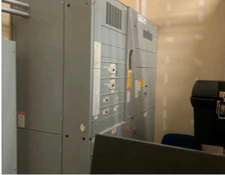
Building Systems - Main Electrical Service
