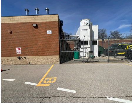
Building Systems - Mechanical System
