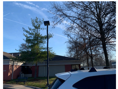
Building Site - Site Lighting
