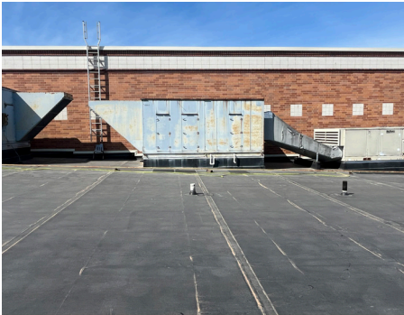
Building Systems - Mechanical System
