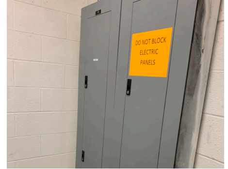
Building Systems - Panelboards
