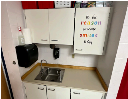
Building Systems - Plumbing Fixtures (Classroom)
