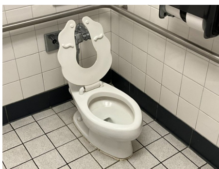
Interior Environment - Plumbing Fixtures
