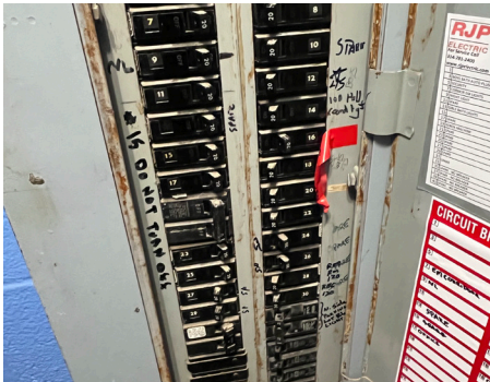
Building Systems - Panelboards
