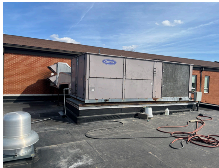
Building Systems - Mechanical System
