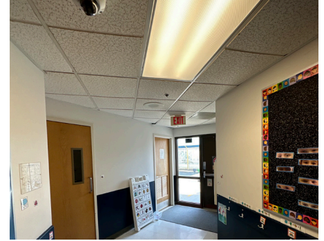
Building Systems - Interior Lighting (Public Areas)
