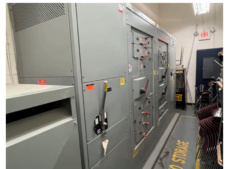
Building Systems - Main Electrical Service
