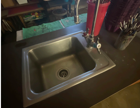
Building Systems - Plumbing Fixtures (Classrooms)
