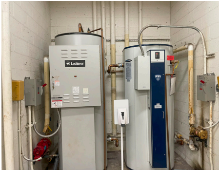
Building Systems - Water Heaters
