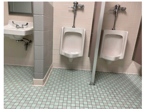
Building Systems - Plumbing Fixtures (Restroom)
