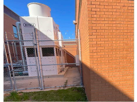
Building Systems - Mechanical System
