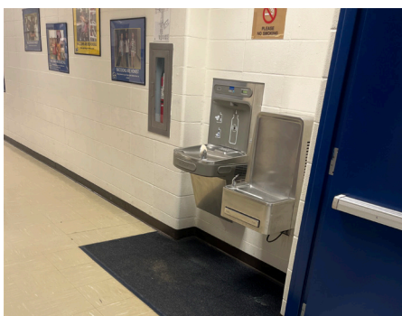
Building Systems - Drinking Fountains
