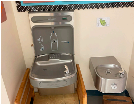
Building Systems - Drinking Fountains
