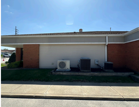
Building Systems - Mechanical System
