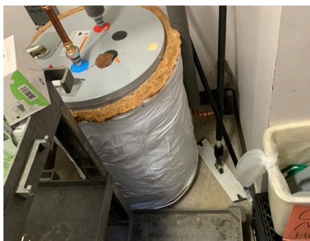
Building Systems - Water Heaters
