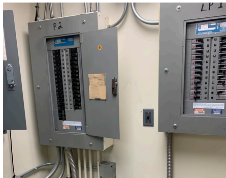
Building System - Panelboards
