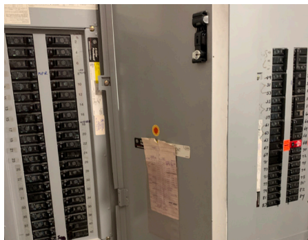
Building Systems - Panelboards
