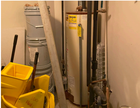
Building Systems - Water Heaters
