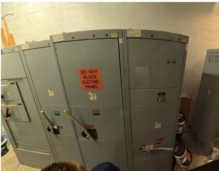
Building Systems - Main Electrical Service
