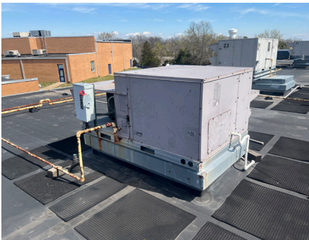
Building Systems - Mechanical System
