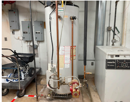
Building Systems - Water Heaters
