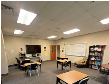
Building Systems - Interior Lighting (Classrooms)
