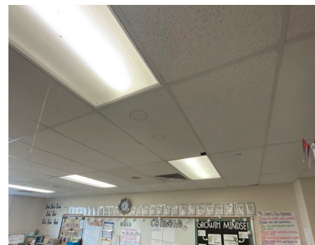
Building Systems - Interior Lighting (Classroom)
