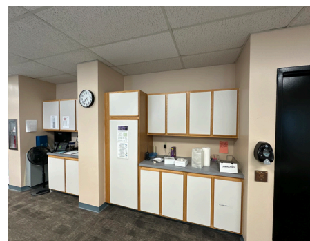
Interior Environment - Casework
