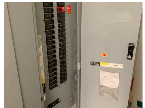
Building Systems - Panelboards
