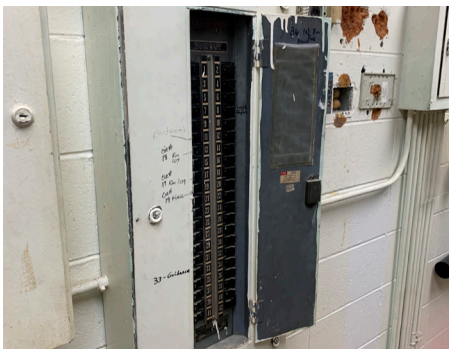
Building Systems - Panelboards
