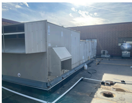
Building Systems - Mechanical Systems
