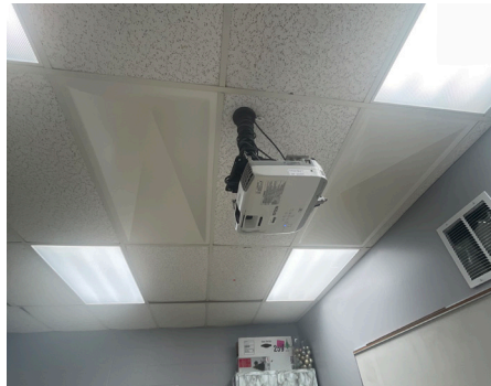
Building Systems - Interior Lighting (Classrooms)
