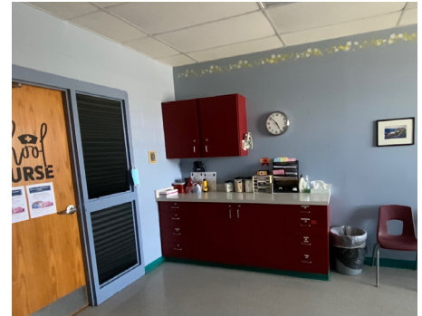
Interior Environment - Casework
