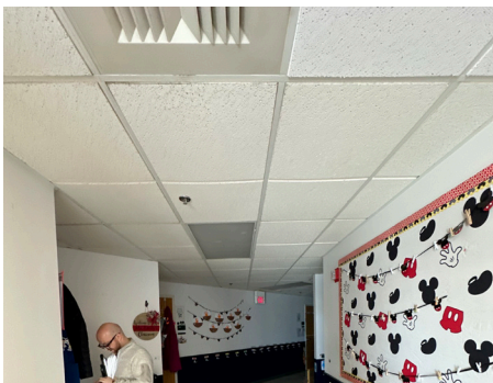
Building Systems - Mechanical System
