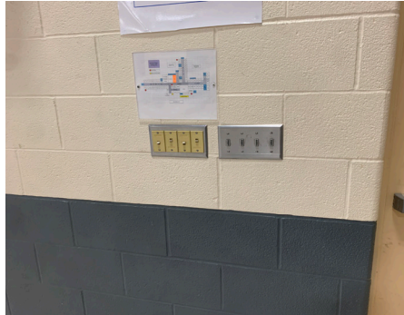
Building Systems - Lighting Controls
