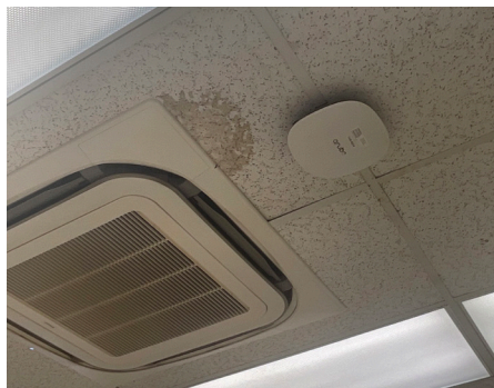
Building Systems - Mechanical Systems
