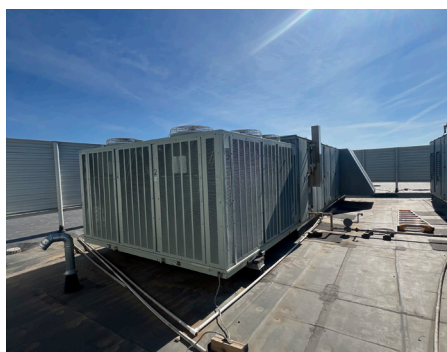
Building Systems - Mechanical System
