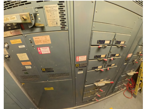
Building Systems - Main Electrical Service
