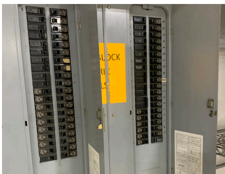
Building Systems - Panelboards
