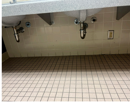
Building Systems - Plumbing Fixtures (Restroom)
