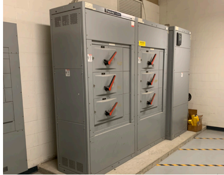
Building Systems - Main Electrical Service
