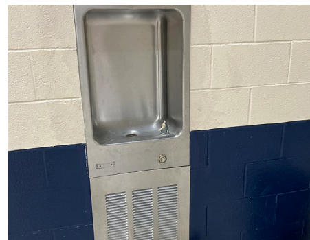
Building Systems - Drinking Fountains
