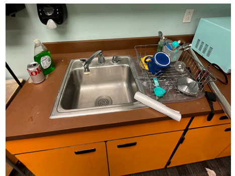
Interior Environment - Casework
