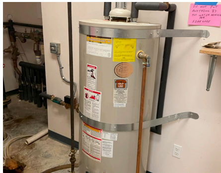
Building Systems - Water Heaters
