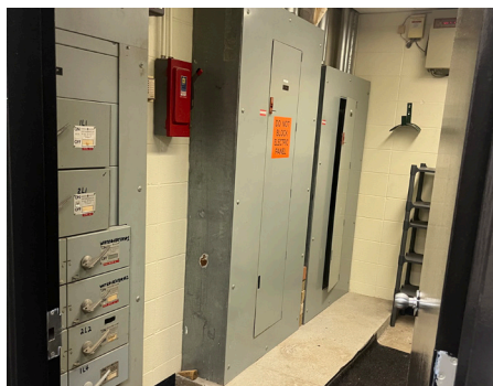
Building Systems - Panelboards
