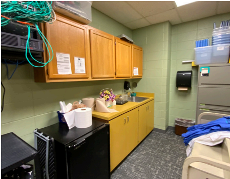
Interior Environment - Casework
