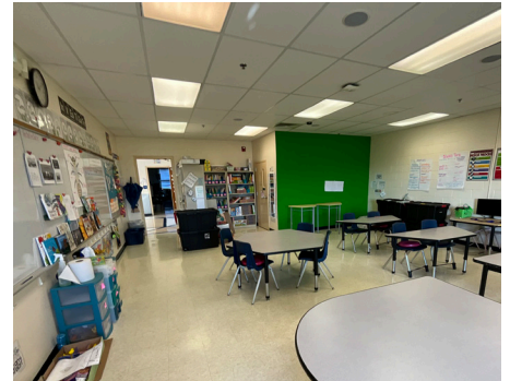
Building Systems - Interior Lighting (Classrooms)
