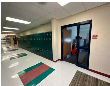
Building Systems - Interior Lighting (Public Areas)
