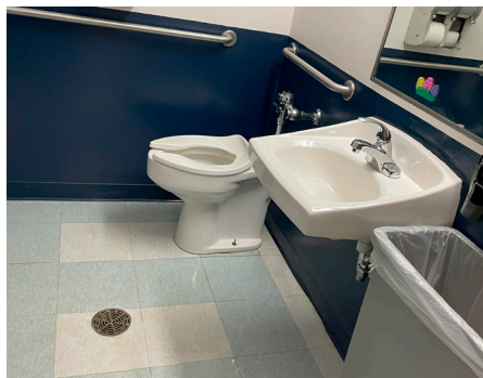
Building Systems - Plumbing Fixtures (Restrooms)
