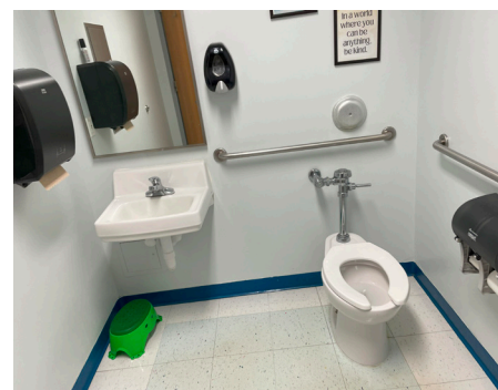
Building Systems - Plumbing Fixtures (Restrooms)
