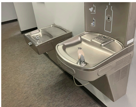
Building Systems - Drinking Fountains
