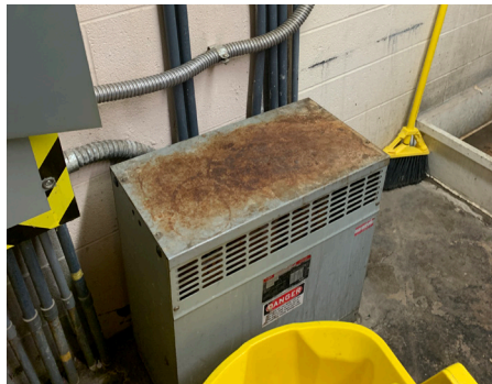
Building Systems - Main Electrical Service
