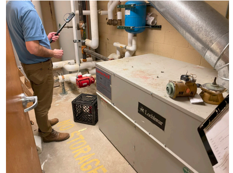
Building System - Water Heaters
