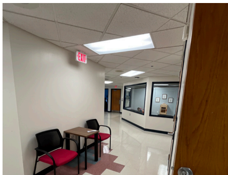
Building Systems - Interior Lighting (Public Areas)
