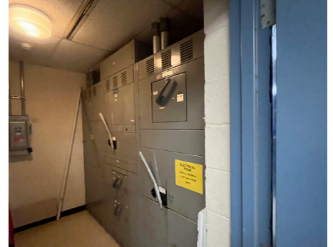
Building Systems - Main Electrical Service
