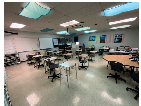
Building Systems - Interior Lighting (Classrooms)
