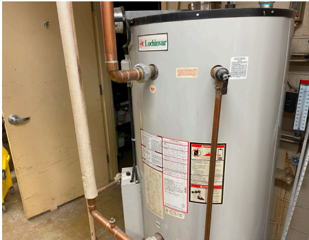
Building Systems - Water Heaters
