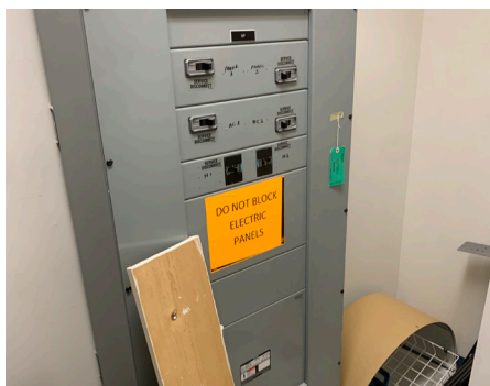
Building Systems - Main Electrical System
