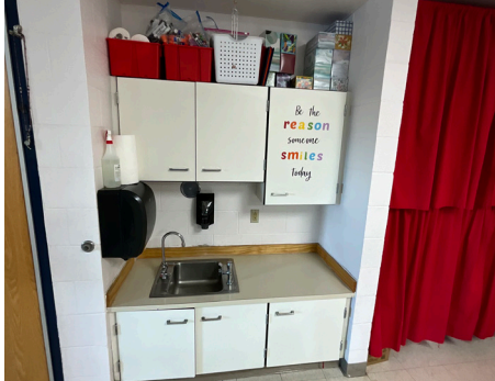
Interior Environment - Casework
