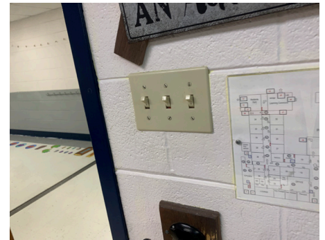
Building Systems - Lighting Controls
