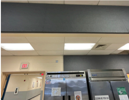
Building Systems - Interior Lighting (Public Areas)
