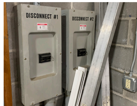
Building Systems - Main Electrical Service
