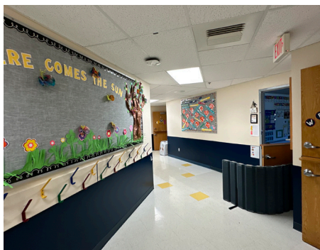
Building Systems - Interior Lighting (Public Areas)
