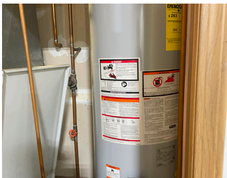
Building Systems - Water Heaters
