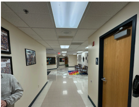
Building Systems - Interior Lighting (Public Areas)
