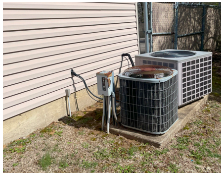
Building Systems - Mechanical System
