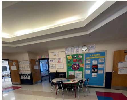
Building Systems - Interior Lighting (Public Areas)
