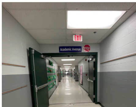
Building Systems - Interior Lighting (Public Areas)
