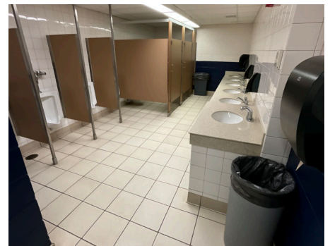
Building Systems - Plumbing Fixtures (Restrooms)
