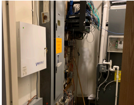
Building Systems - Main Electrical Service
