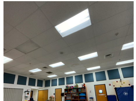
Building Systems - Interior Lighting (Classrooms)
