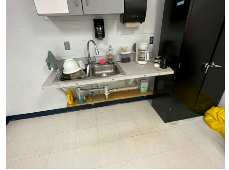
Interior Environment - Plumbing Fixtures
