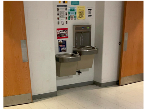
Building Systems - Drinking Fountains
