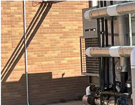
Building Systems - Mechanical System
