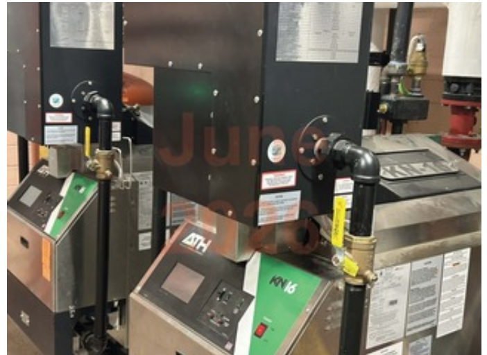
New Boiler (2026 Photo)
