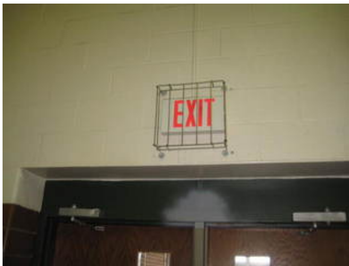
Illuminated Exit Sign
