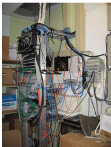
OSDM Non-Compliant Computer Network Infrastructure
