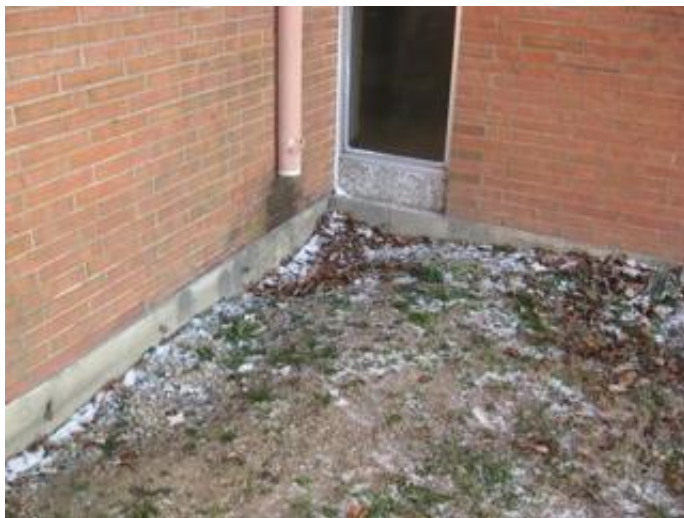
Condition of Grade at Foundation and Roof Drain Location
