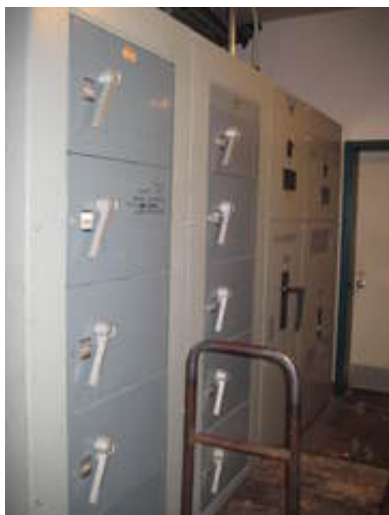
Main Electrical Distribution Panel
