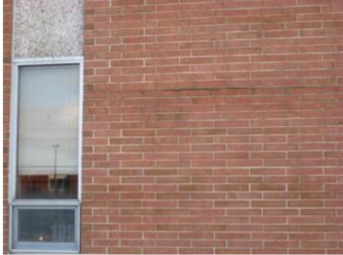
Horizontal Joint Cracking in Exterior Masonry
