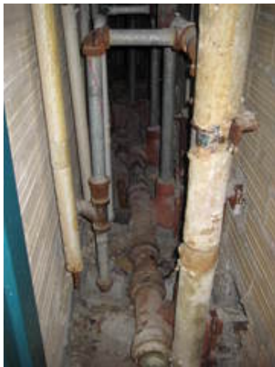
Sanitary Waste Piping
