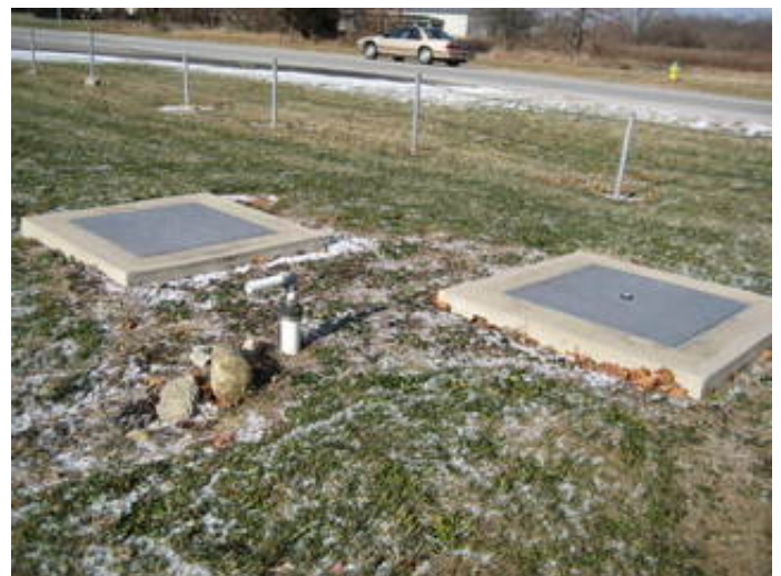
Incoming Domestic Water Meter Pits
