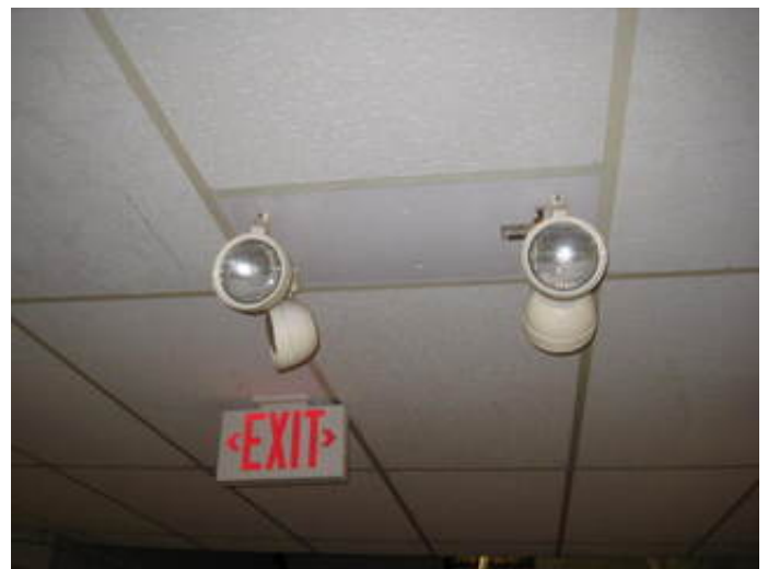
Emergency Egress Light Fixture
