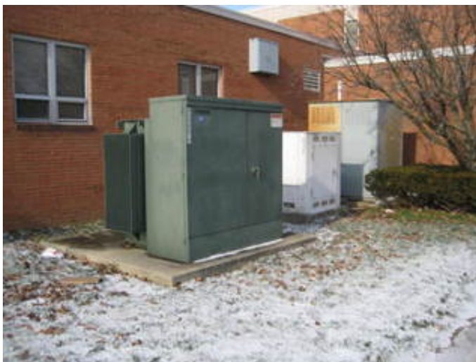
Pad Mounted Transformer
