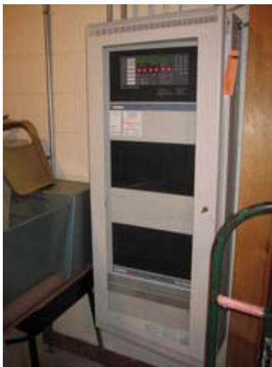
Fire Alarm System Control Panel
