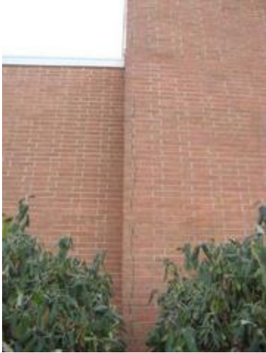
Masonry Cracks at Building Offset
