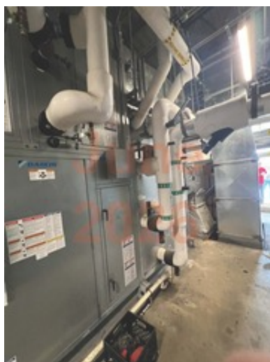
New HVAC Units (2026 Photo)
