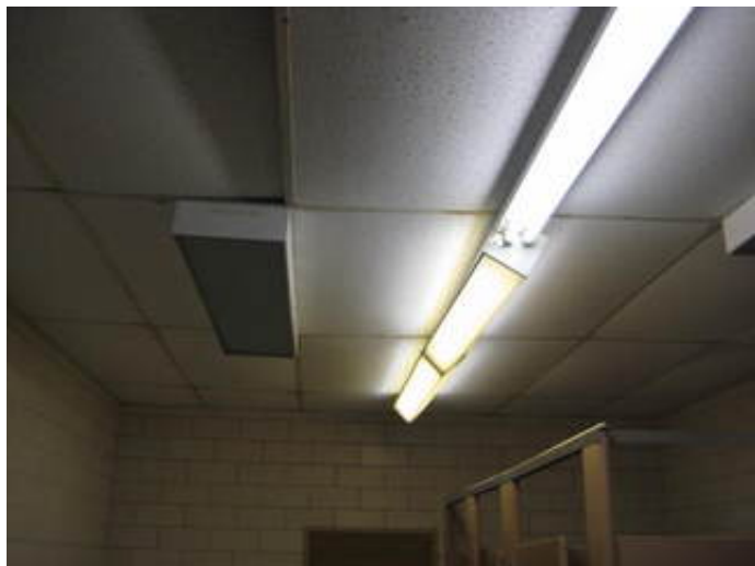
Surface Mounted Fluorescent Light Fixtures
