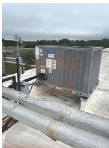
Rooftop Unit (2026 Photo)
