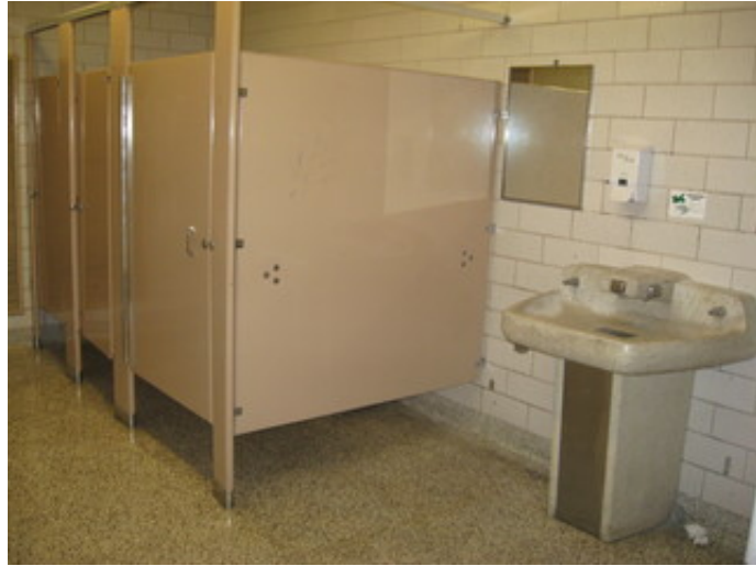
Typical Boy's Restroom With Non-Compliant ADA Toilet Stall
