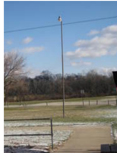
Pole-mounted LED light fixture (formerly HID high-pressure sodium)
