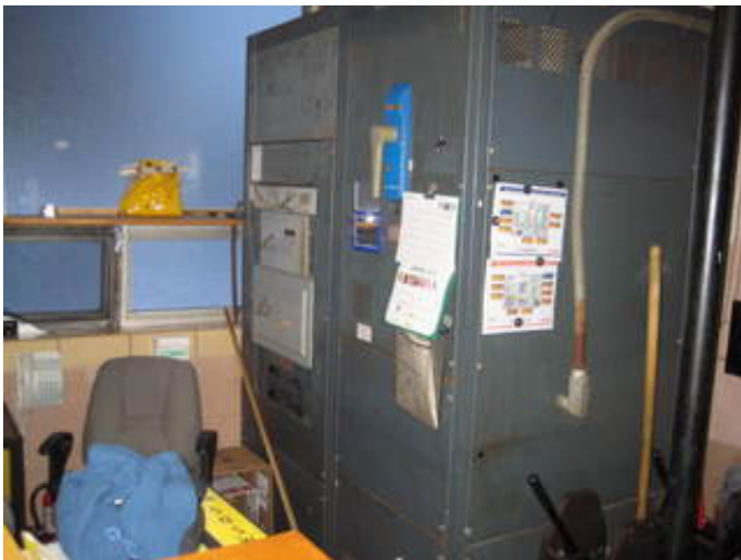
Main Electrical Distribution Panel
