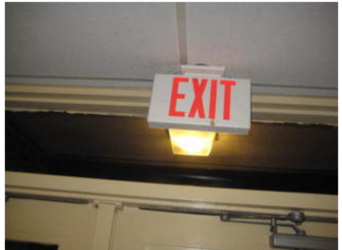
Non-compliant Exit Sign
