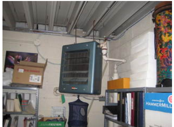
Heating Water Unit Heater
