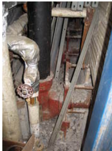
Sanitary Waste Piping
