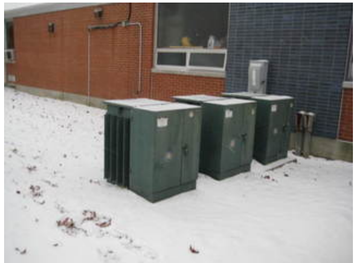
Pad Mounted Transformers
