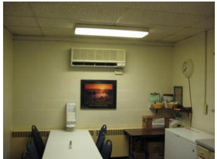
Teacher's Lounge Ductless Split AC Unit
