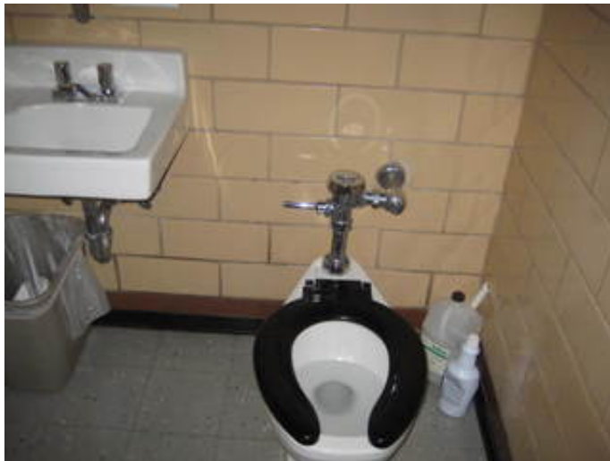
Non-ADA Wall Hung Lavatory and Floor Mounted Flush Valve Toilet
