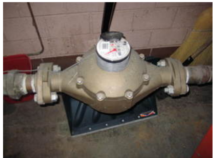
Incoming Domestic Water Service Meter
