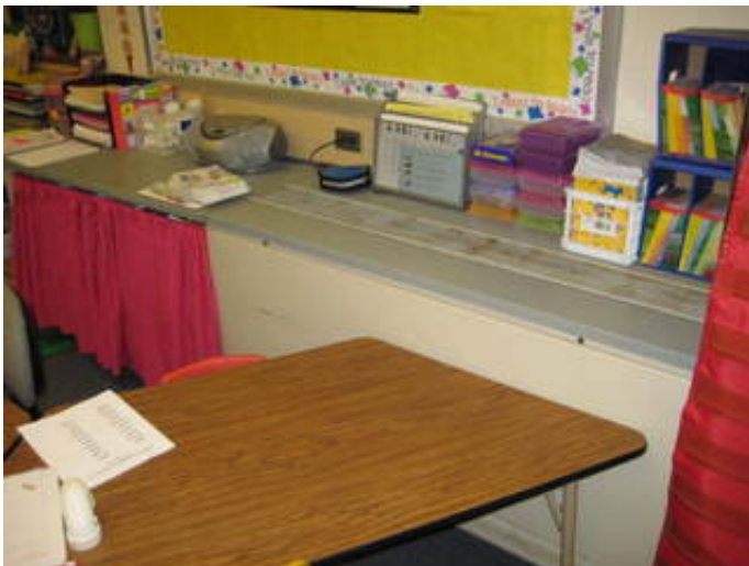
Typical Classroom Unit Ventilator
