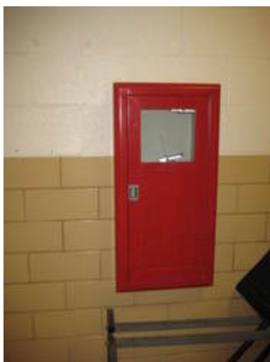
Wall Cabinet and Fire Extinguisher
