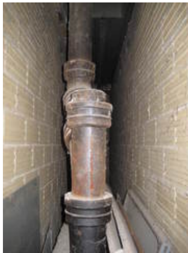
Sanitary Waste Piping
