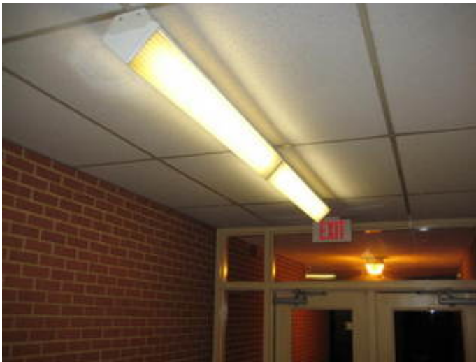
Typical Corridor Fluorescent Light Fixture
