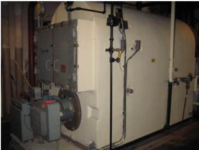
Natural Gas Fired Heated Water Boiler
