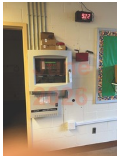
Fire Alarm System Control Panel (2026 Photo)
