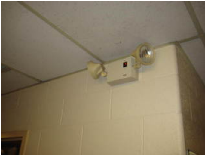
Emergency Egress Light Fixture
