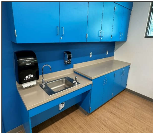
Kindergarten Classroom Cabinet/Sink
