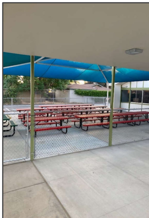
New Electrical Service
