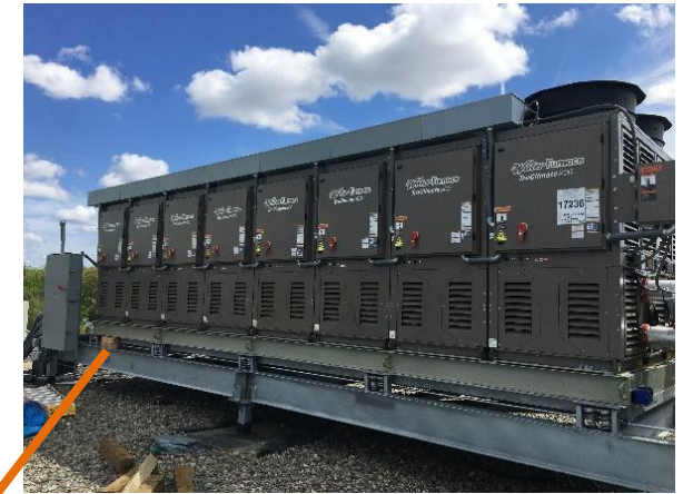
Central ASHP recently installed at Newton Library
