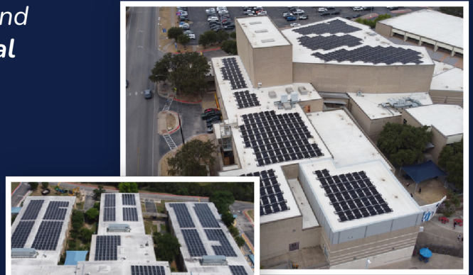
Solar panels at BCE & WHS
