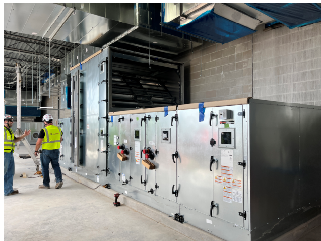
HVAC Equipment – Area B1 Pool Mechanical Room
