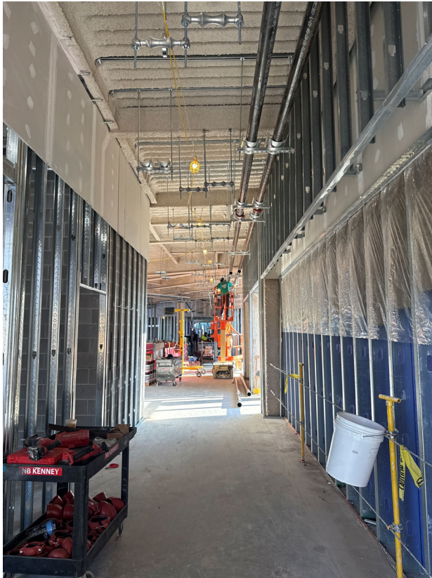
Overhead MEP's, Building B East (near bridge)
