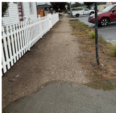
Figure 8. Missing sidewalk on Purissima St.
