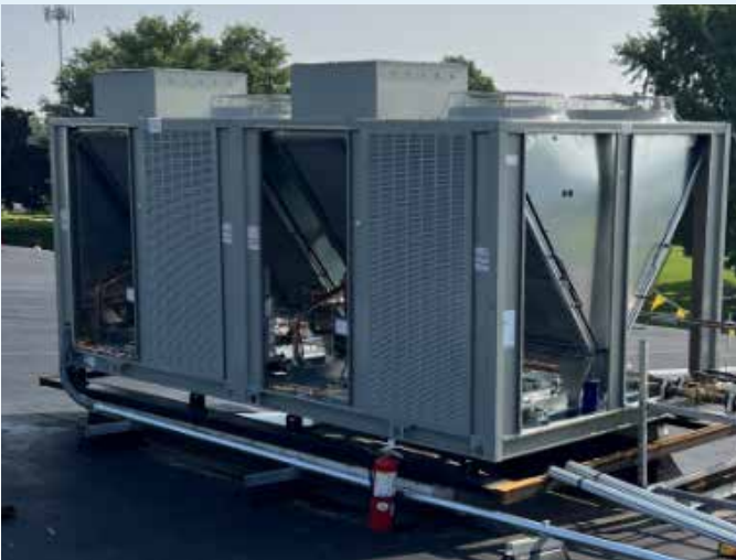
New HVAC System at Black Hawk Elementary.
